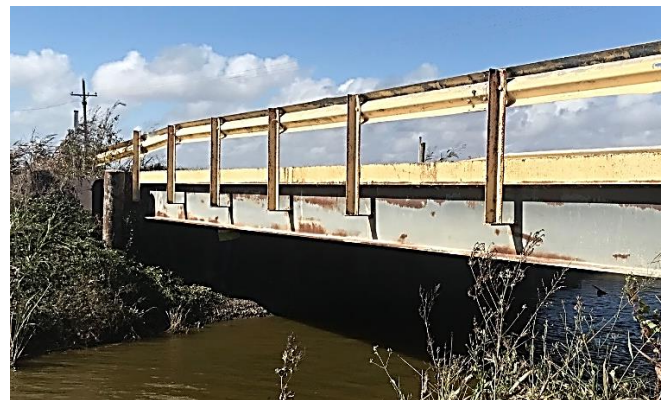
Figure 3. Corrosion on Painted Steel Girder.
