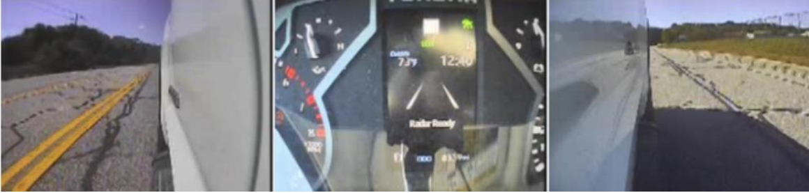
Figure 4-14: Elements of Pavement Repair that are Perceived as Markings by ADAS.
