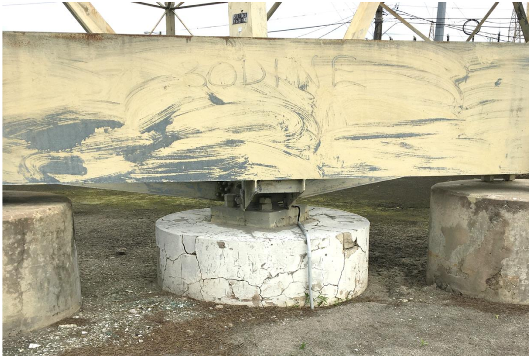
Figure 1.1 Example of a damaged drilled shaft.
