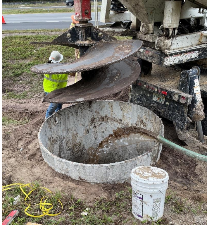
Figure 3.28 Excavation of drilled shaft OC-19 with partial-length casing installed. [This is a photo showing the construction location of drilled shaft OC-19. The location is still in the process of being augered with slurry flowing from a large hose line. The partial-length casing is already placed inside the augered portion.]
