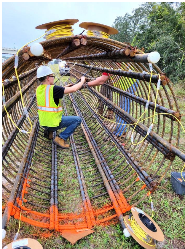
Figure 3.29 Installation of thermal wires along the length of the OC-19 reinforcement cage. [This is a photo taken from the top of the OC-19 reinforcement cage showing installed cage thermal wires positioned roughly 90 degrees apart radially.]
