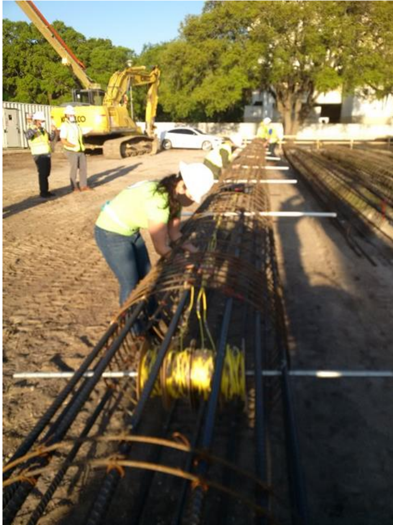
Figure 1.7 Installation of thermal wires to a shaft reinforcing cage at a construction site located on the University of South Florida Tampa Campus.
