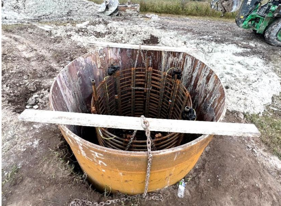
Figure 3.20 Fully instrumented OC-13 reinforcement cage placed in the augered location prior to concrete placement.
