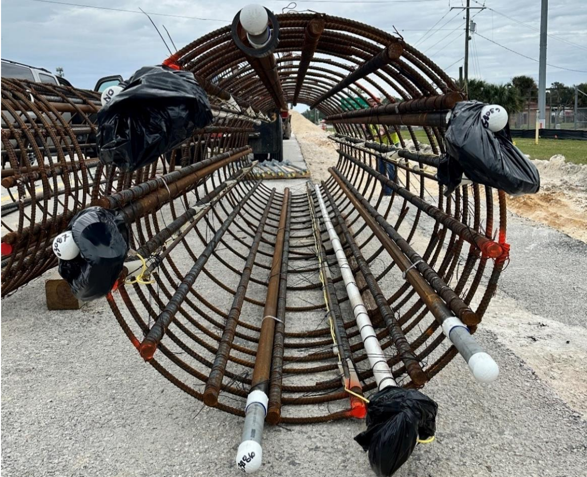
Figure 3.58 Fully instrumented Bartow shaft 1-4 reinforcement cage ready to be placed for concrete casting.
