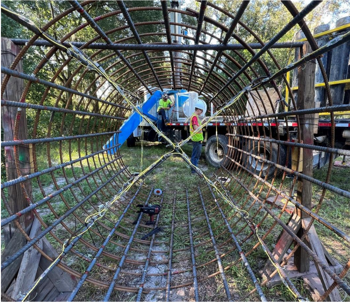
Figure 3.48 Complete installation of center thermal wire inside Sinclair Hills drilled shaft reinforcement cage.
