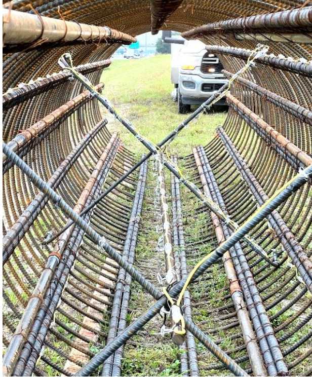
Figure 3.31 Complete installation of center thermal wire inside OC-19 reinforcement cage. [This is a photo taken inside the OC-19 reinforcement cage showing center thermal wire installation including across shaft sensor configuration. The bottom 15 thermal sensors are shown to be installed on three out of four legs of the bottom cross bracing.]
