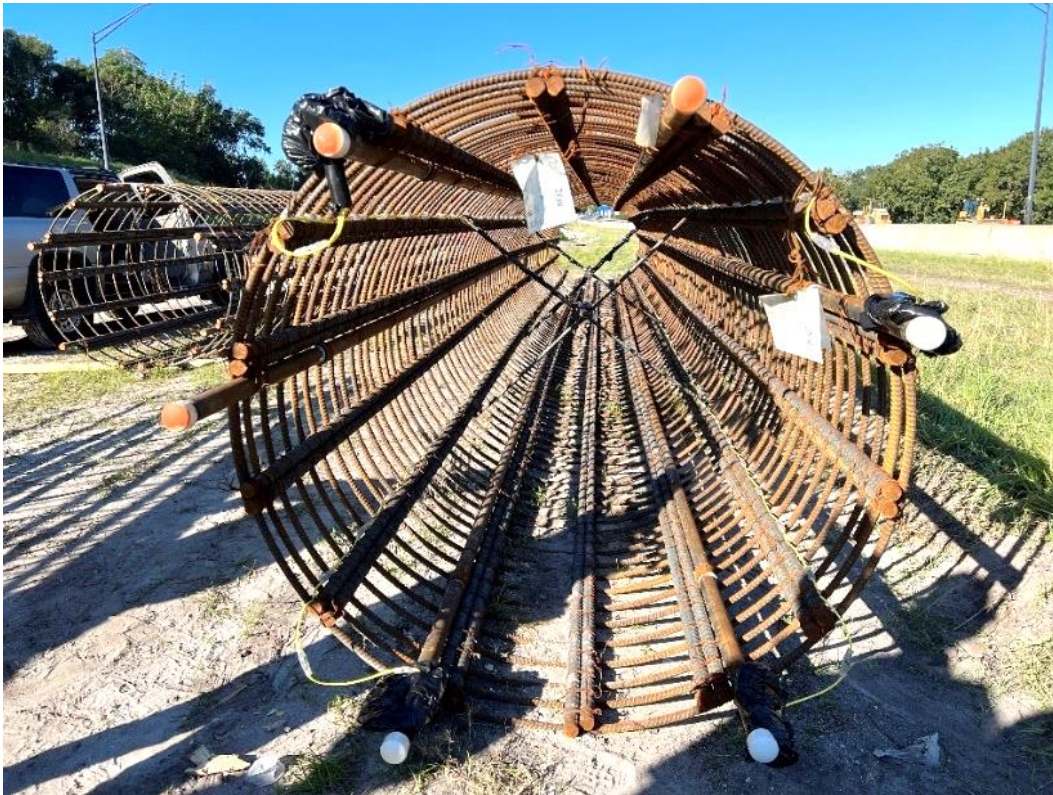
Figure 3.19 Fully instrumented OC-13 reinforcement cage ready to be placed for concrete casting. [This is a photo taken from outside the top of the OC-13 reinforcement cage. All cage thermal wires and center thermal wire have been installed, and all above-concrete sensors and wire connector ends have been bundled and secured in heavy-duty plastic bags and Gorilla tape.]
