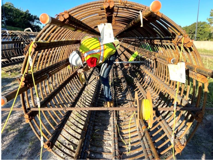
Figure 3.15 Installation of thermal wires along the length of the OC-13 reinforcement cage. [This is a photo taken from the top of the OC-13 reinforcement cage showing installed cage thermal wires positioned roughly 90 degrees apart radially.]
