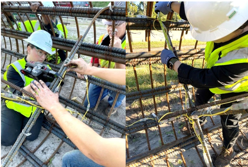
Figure 3.18 Installation of the bottom 15 sensors of the center thermal wire in an across-shaft configuration along the bottom rebar cross bracing in OC-13 reinforcement cage.
