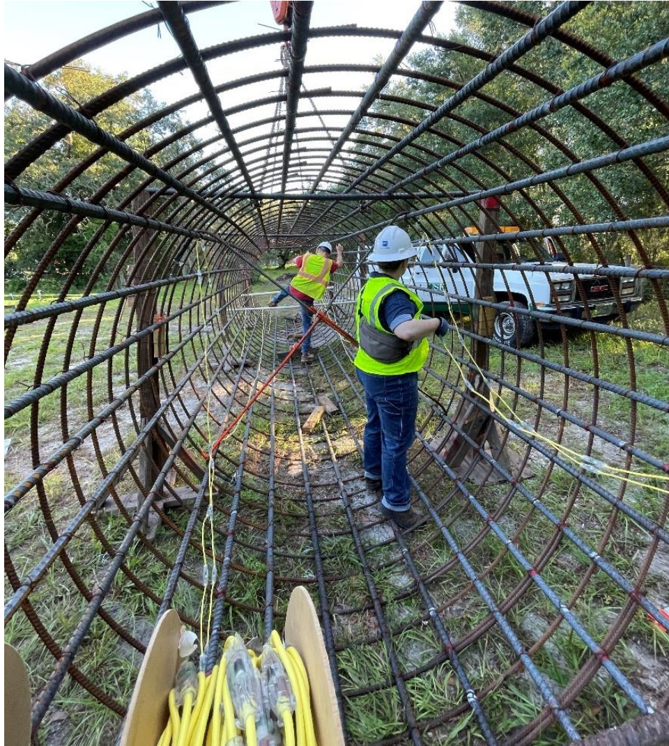
Figure 3.46 Installation of thermal wires along the length of the Sinclair Hills drilled shaft reinforcement cage.
