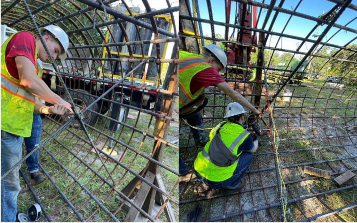
Figure 3.47 Installation of the rebar cross bracing and the center thermal wire in an across-shaft configuration along the rebar cross bracing.
