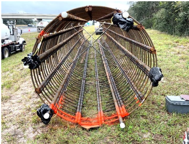
Figure 3.32 Fully instrumented OC-19 reinforcement cage ready to be placed for concrete casting. [This is a photo taken from outside the top of the OC-19 reinforcement cage. All cage thermal wires and center thermal wire have been installed, and all above-concrete sensors and wire connector ends have been bundled and secured in heavy-duty plastic bags and Gorilla tape.]
