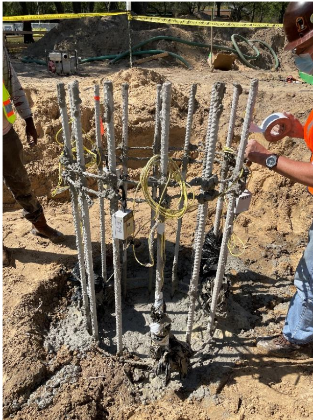
Figure 3.5 Connection of the Thermal Acquisition Port boxes after concrete placement. [This is a photo of DS-6 after concrete placement with approximately five feet of rebar stick-up illustrating the connection of Thermal Acquisition Port boxes to the thermal wires to begin data collection.]
