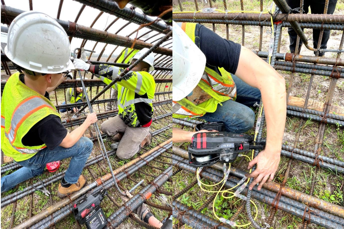
Figure 3.30 Installation of the center rebar cross bracing and the bottom 15 sensors of the center thermal wire in an across-shaft configuration along the bottom rebar cross bracing in OC-19 reinforcement cage.
