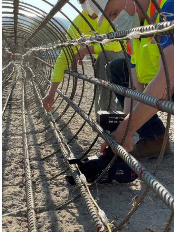
Figure 3.2 Installation of thermal wires along the length of the DS-6 reinforcement cage. [This is a photo taken from inside the DS-6 reinforcement cage showing a completely installed thermal wire at the top right and an in process thermal wire installation at the bottom right.]
