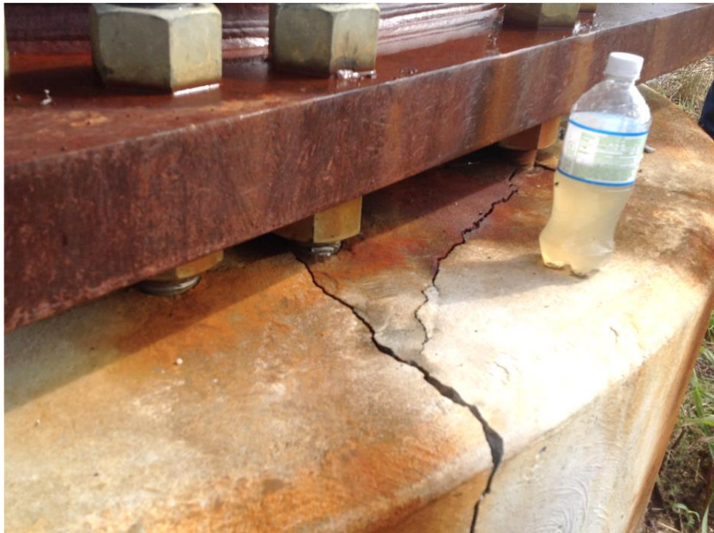
Figure 1.2 Temperature-induced damage to drilled shaft (courtesy of Chris Harris with R.W. Harris, Inc.).
