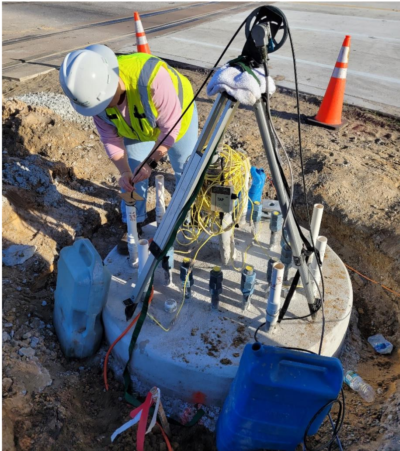
Figure 4.32 Thermal integrity probe test performed on Bartow shaft 1-4 with gyroscopic sensor. [This is a photograph of a graduate student taking probe temperature measurements using a thermal probe equipped with a gyroscopic sensor. The graduate student is seen rotating the probe within the access tube.]
