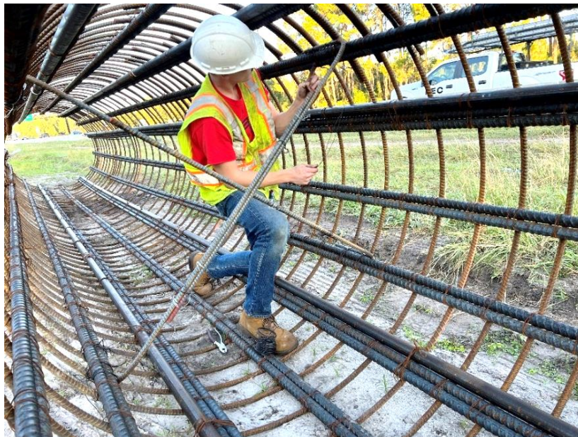
Figure 3.16 Installation of the center rebar cross bracing for drilled shaft OC-13. [This is a photo taken from inside the OC-13 reinforcement cage showing a graduate student securing the cross bracing that will be used to secure the center rebar for the center thermal wire.]
