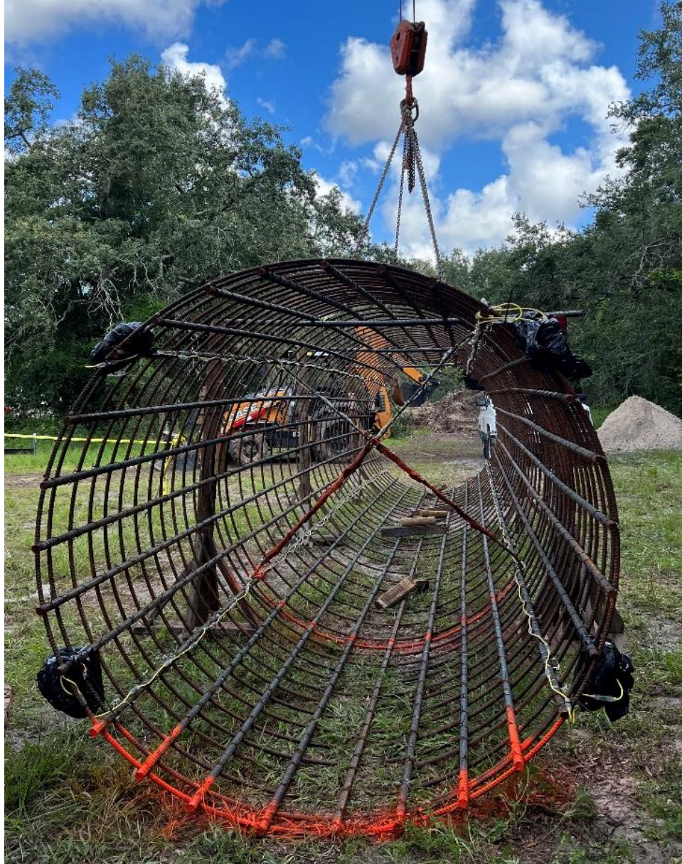
Figure 3.49 Fully instrumented Sinclair Hills drilled shaft reinforcement cage ready to be placed for concrete casting.
