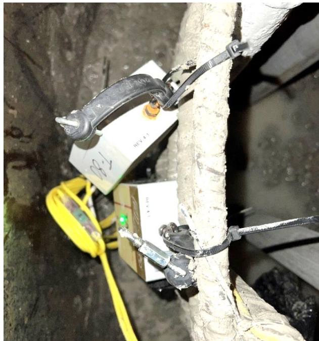
Figure 3.21 Two out of five total OC-13 TAP boxes connected to their respective thermal wires.
