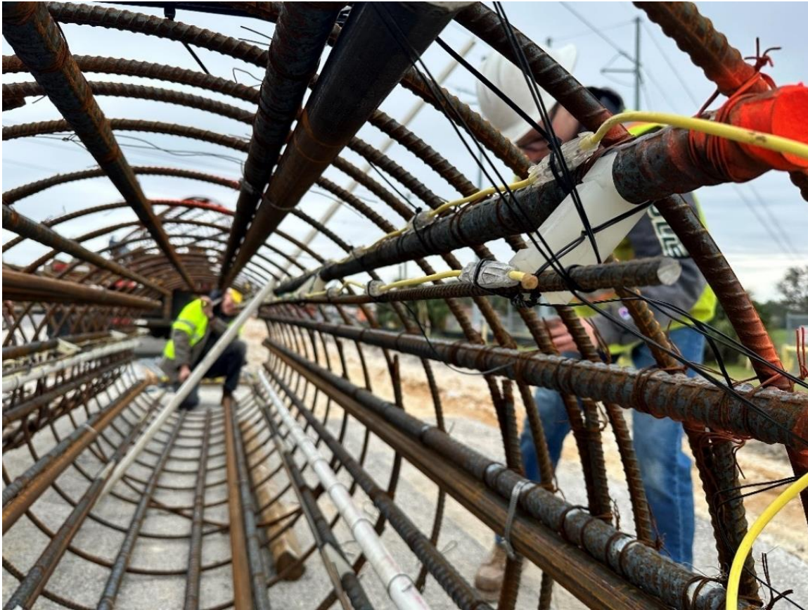
Figure 3.57 Close up view of thermal wire installed at the reinforcement cage with offset return wire.
