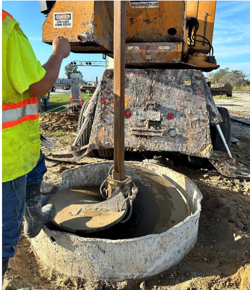
Figure 3.56 Partially augered location of Bartow shaft 1-4 with partial-length casing installed. [This is a photo showing the construction location of the Bartow drilled shaft. The location is still in the process of being augered. The partial-length casing is already placed inside the augered portion.]
