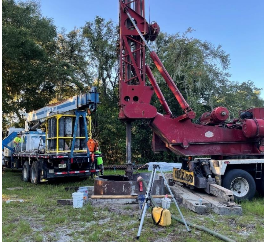
Figure 3.45 Excavation of the Sinclair Hills drilled shaft with partial-length casing installed. [This is a photo showing the construction location of the Sinclair Hills drilled shaft. The location is still in the process of being augered with slurry flowing from a large hose line. The partial-length casing is already placed inside the augered portion.]
