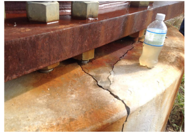
A drilled shaft exhibits large temperature-induced surface cracks.
