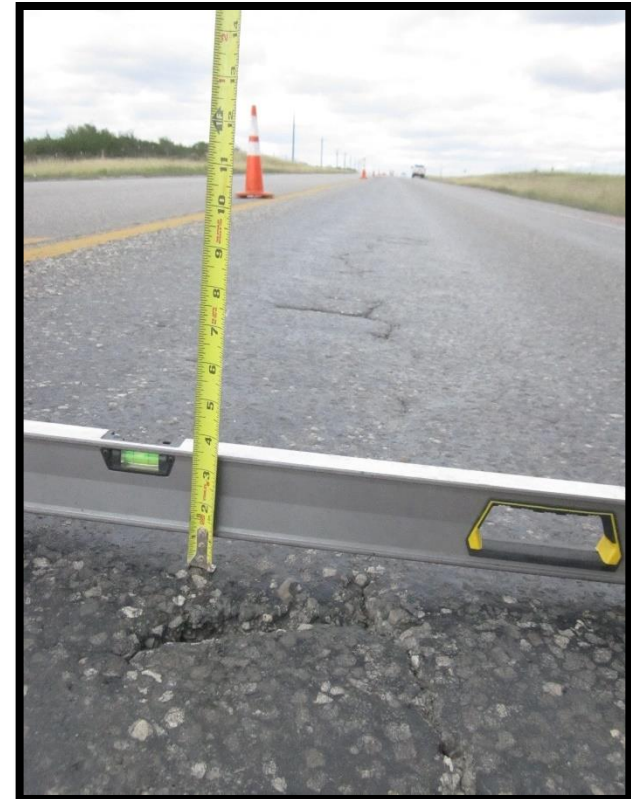
Wide, deep rutting suggests triaxial failure
