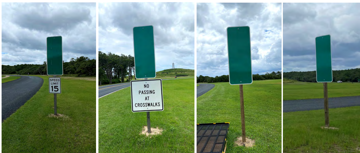
Figure 28: The Four Localization Signs Installed Along Shuttle's Route
