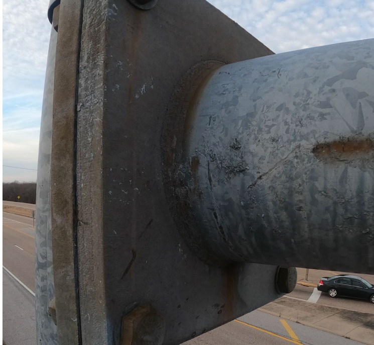
Figure 86. Photo. Example welded aerial connection in poor condition.
