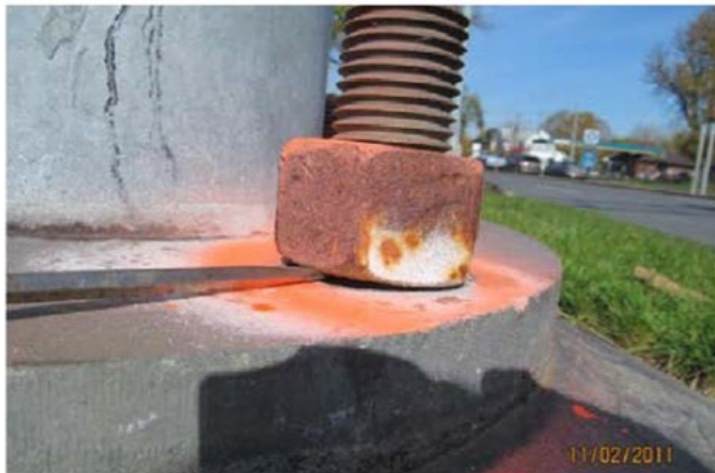
Figure 79. Photo. Example of foundation and base plate connection in poor condition.
