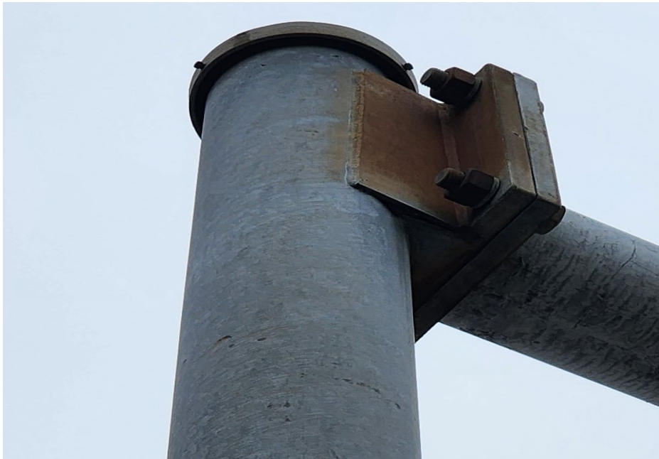
Figure 83. Photo. Example of bolted aerial connection in poor condition.
