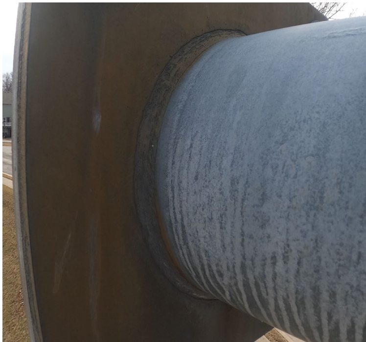
Figure 87. Photo. Example welded aerial connection in good condition.
