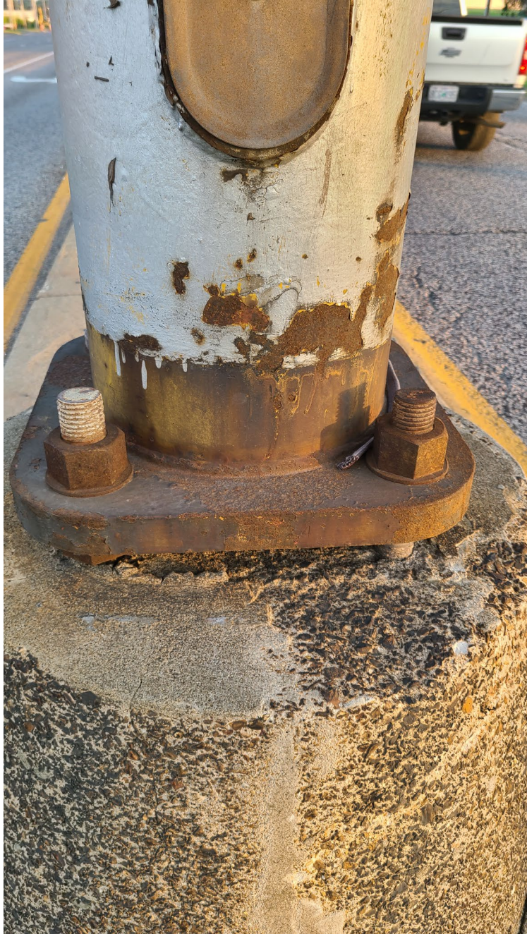
Figure 96. Photo. Example of a base plate and pole in critical condition.
