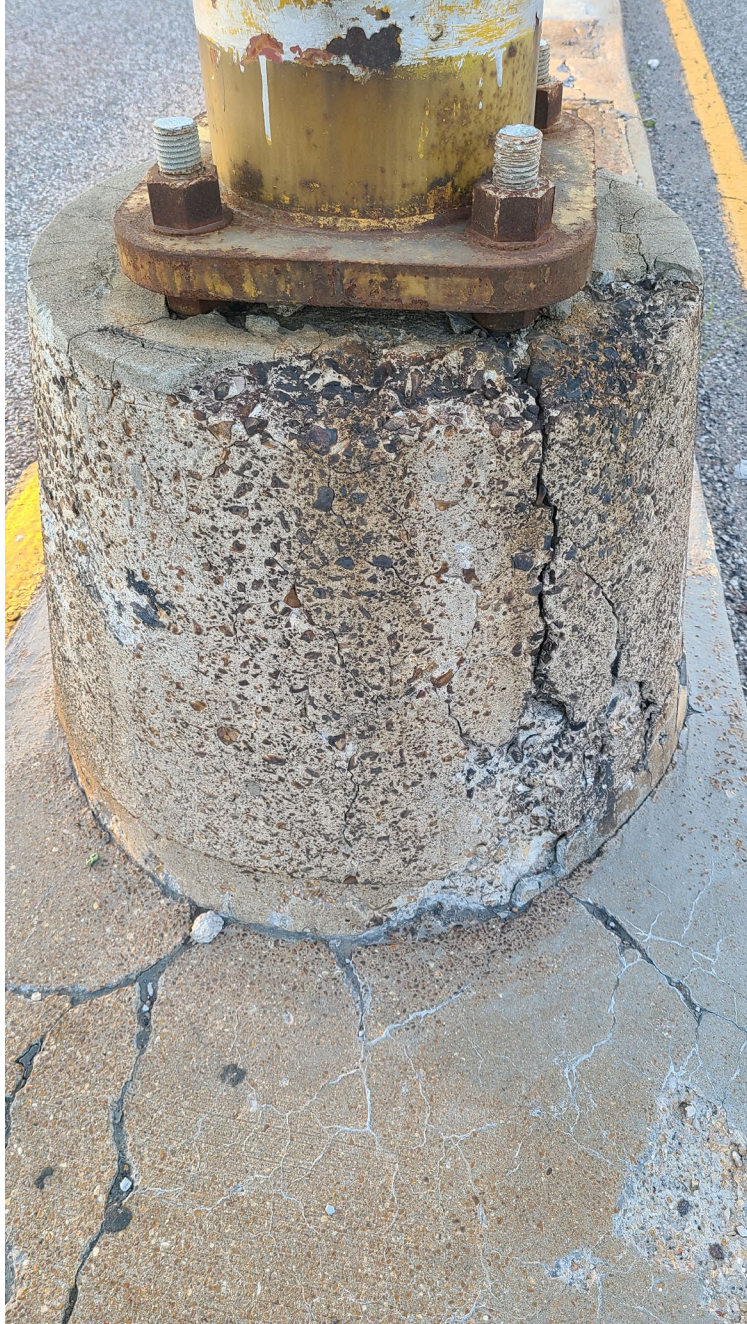
Figure 97. Photo. Example of a base in critical condition.
