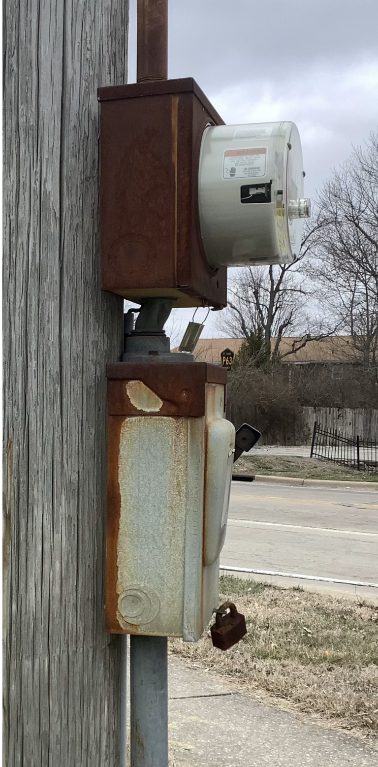
Figure 94. Photo. Example of a power service in poor condition.
