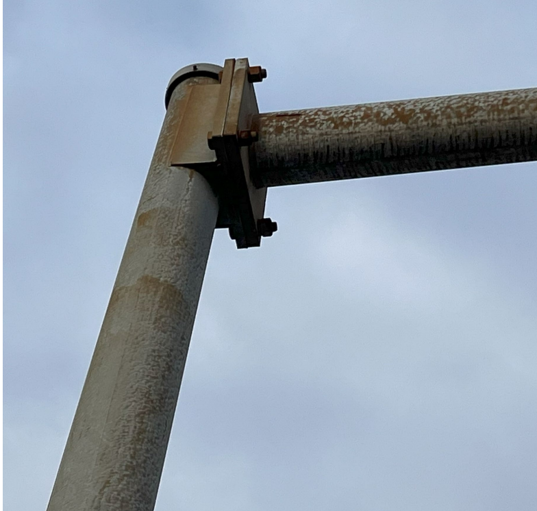
Figure 84. Photo. Example of a bolted aerial connection in critical condition.
