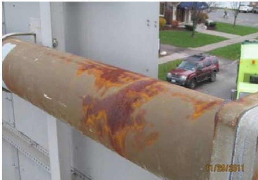
Figure 93. Photo. Example of mast arm in poor condition.
