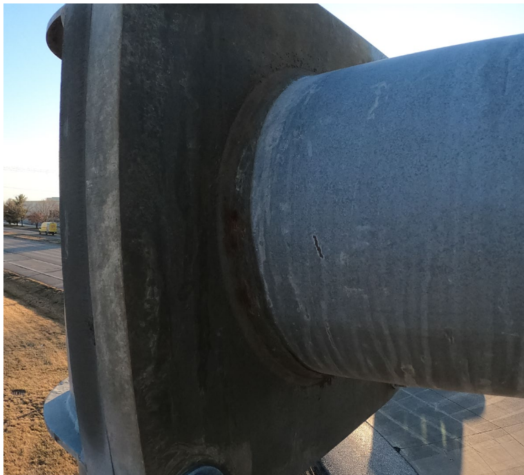
Figure 85. Photo. Example welded aerial connection in fair condition.
