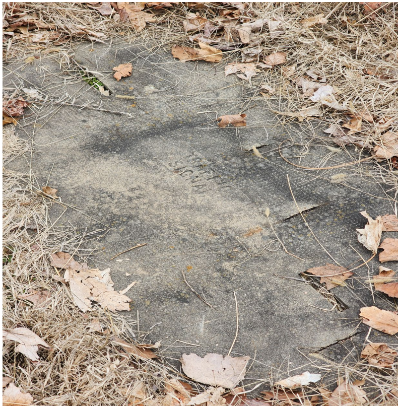
Figure 81. Photo. Example junction box in poor condition.
