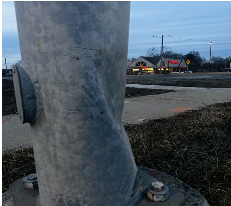
Figure 91. Photo. Example pole dent in critical condition.
