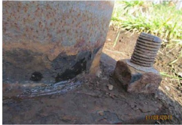
Figure 76. Photo. Example of base plate coating in critical condition.
