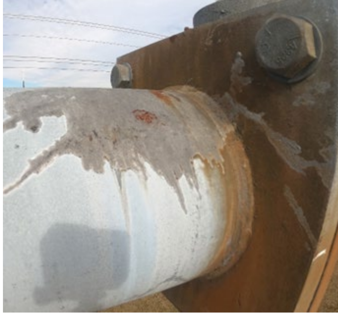
Figure 88. Photo. Example welded connection in critical condition.
