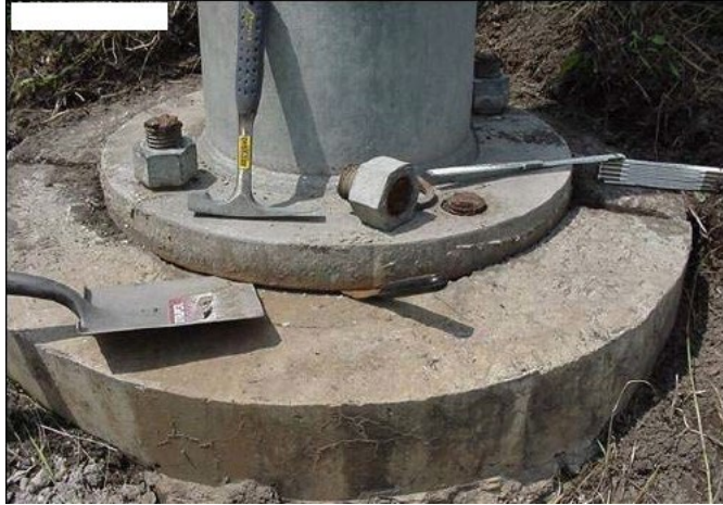
Figure 80. Photo. Example of foundation and base plate connection in critical condition.
