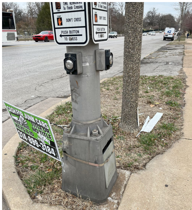
Figure 77. Photo. Example of transformer base in critical condition.
