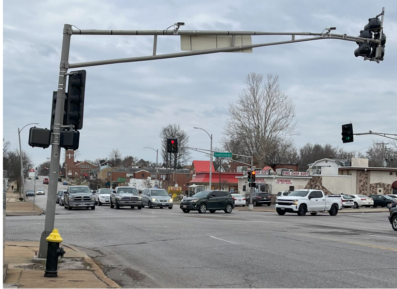
Figure 90. Photo. Example of pole plumbness in critical condition.
