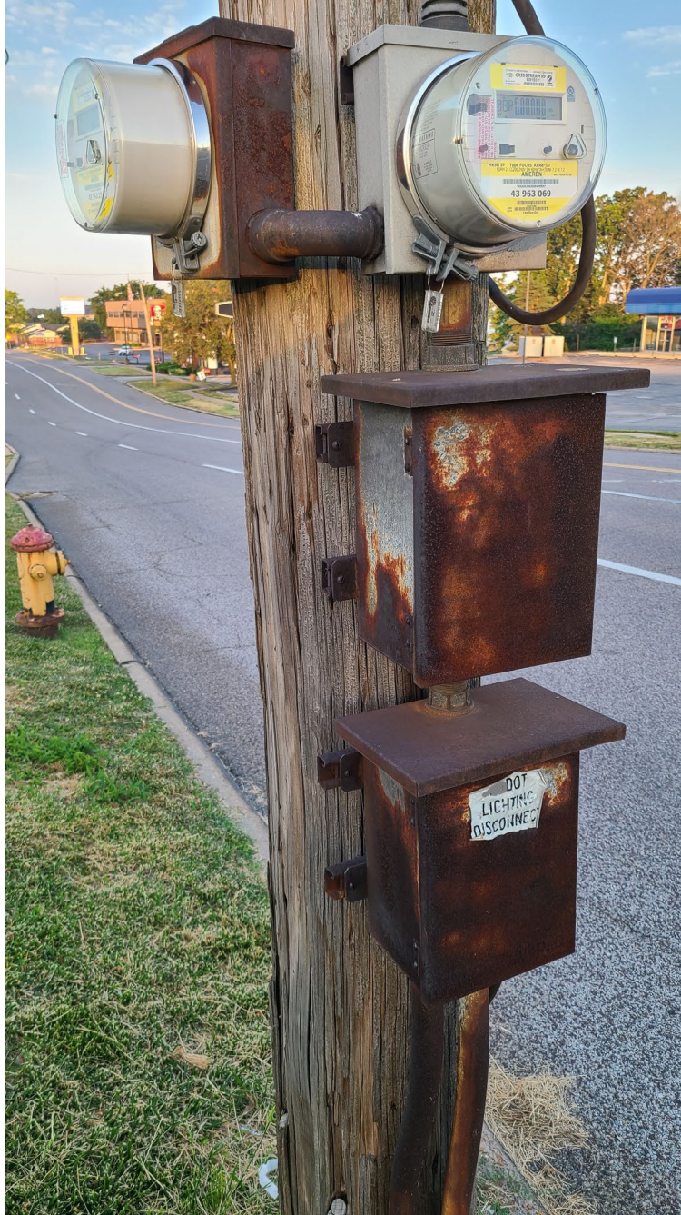
Figure 95. Photo. Example of a power service in critical condition.
