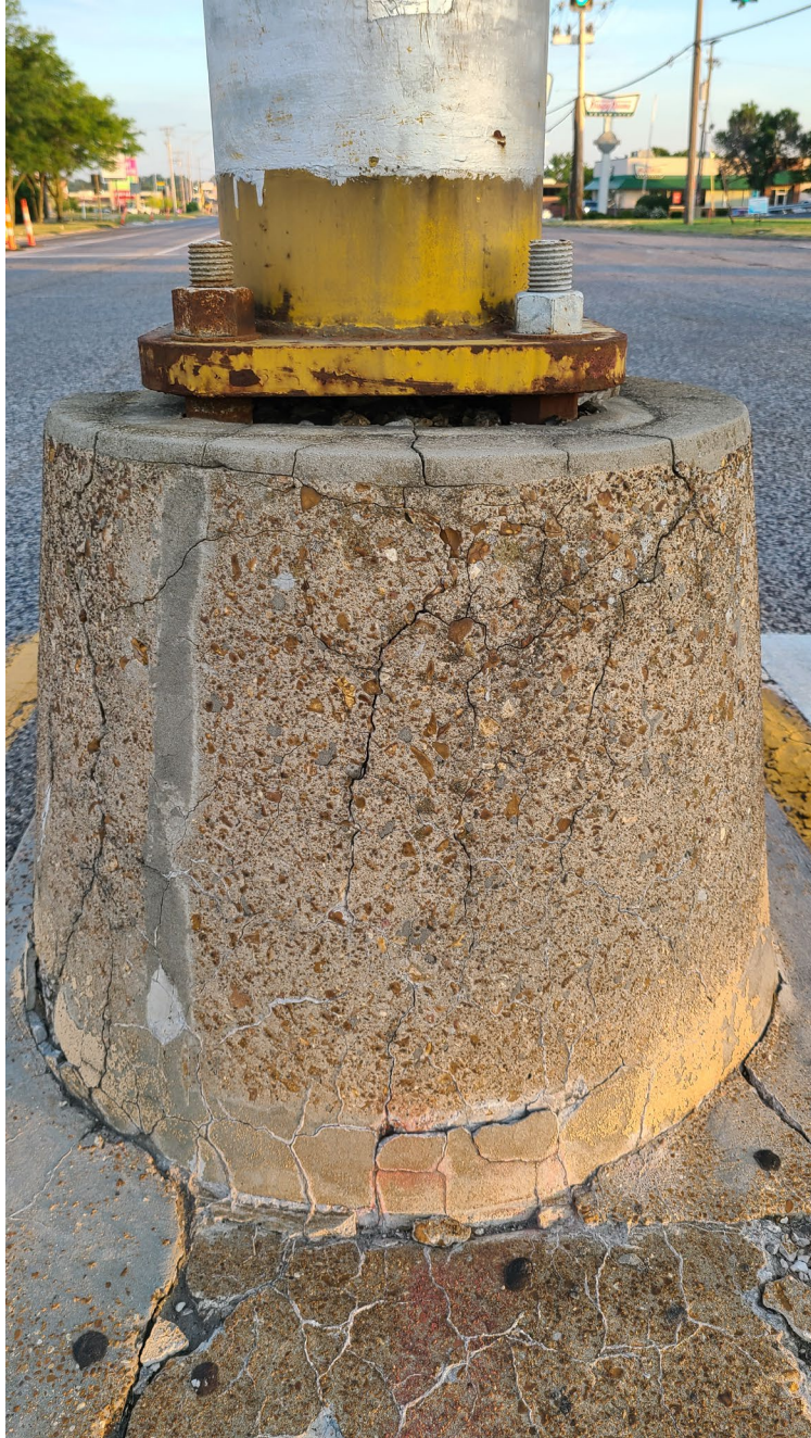
Figure 98. Photo. Example of a base in poor condition.
