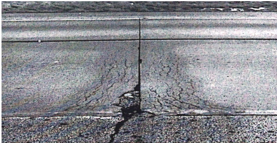
Figure 2.4: Development of D-Cracking Along Joints
