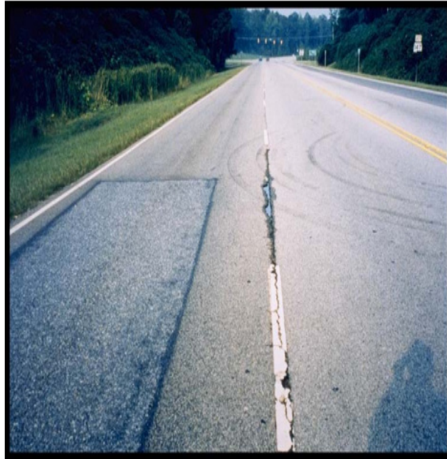
Figure 2.4: Opening of longitudinal joint. (Brown 2016)
