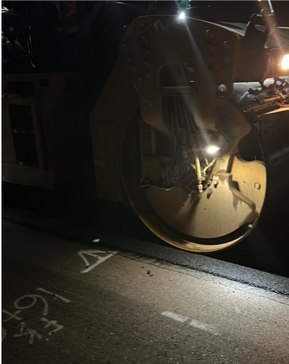
Figure 5.5: Hot Pinch construction with roller 152mm away from the longitudinal joint – I5-Kuebler, 08/17/2023.
