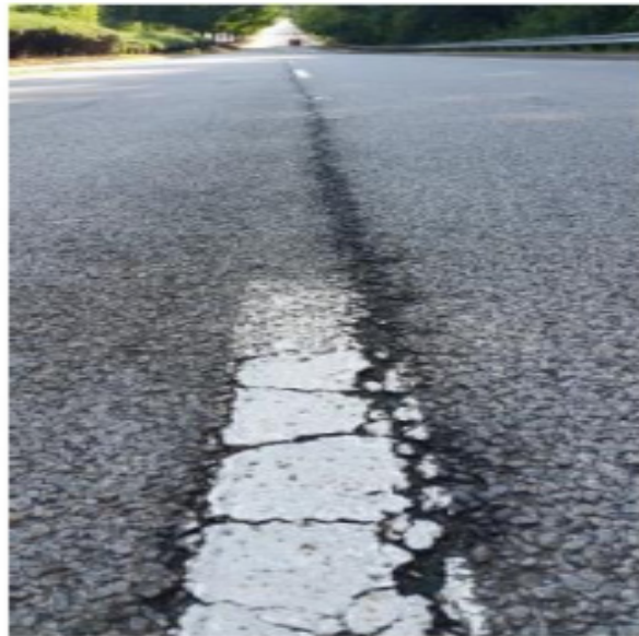
Figure 2.5: Cracking at the longitudinal joint. (Kim 2017)
