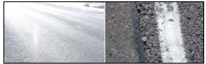
Figure 8. Transverse cracking (left) and longitudinal edge cracking (right). (Source: Musa Ruranika and Geib)
