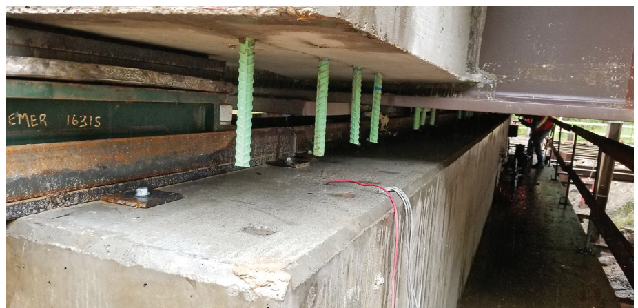
Closure joint between super- and sub-structure during the construction of a multi-span bridge using SIBC on IA 1 over Old Man's Creek southwest of Iowa City
