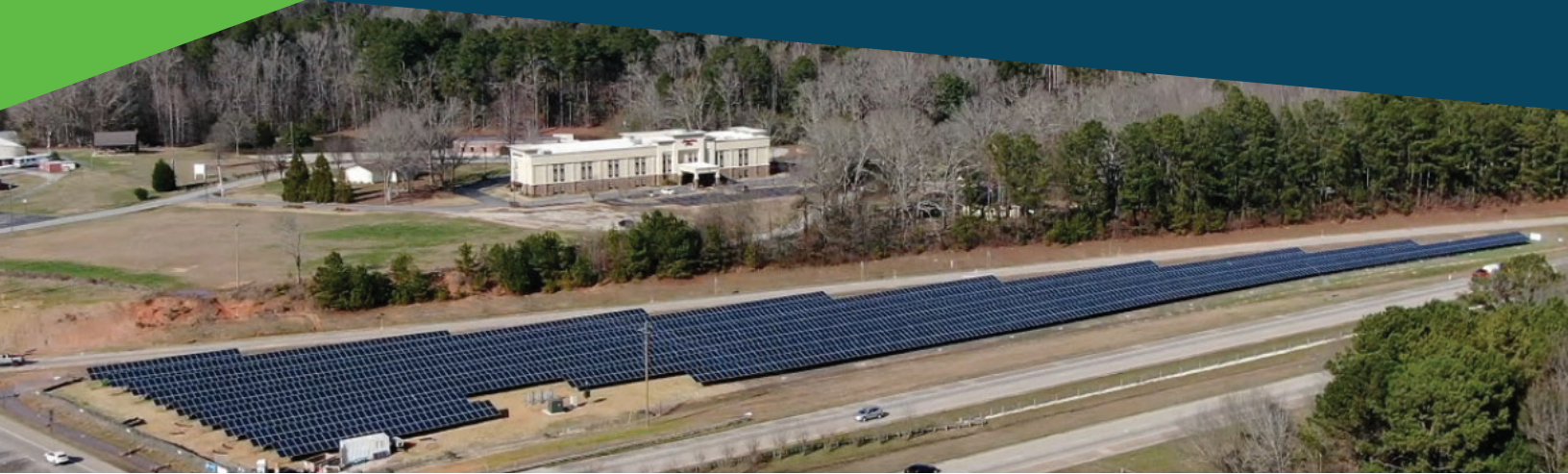
Figure 15: Solar array on I-85 developed by Georgia Power on Georgia DOT right-of-way. (Photo credit: The Ray).
