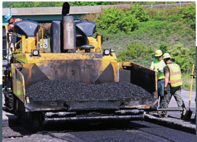
Figure 14: Using warm mix asphalt instead of standard practices produces 37 percent lower GHG emissions, according to FHWA's Infrastructure Carbon Estimator. (Photo credit: PennDOT).
