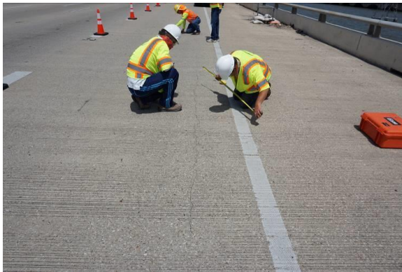
Longitudinal crack on Bridge Deck #9
