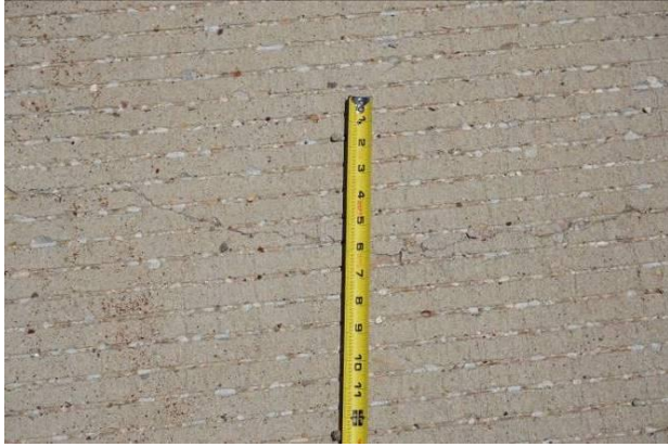
Transverse Cracks on Bridge Deck #6
