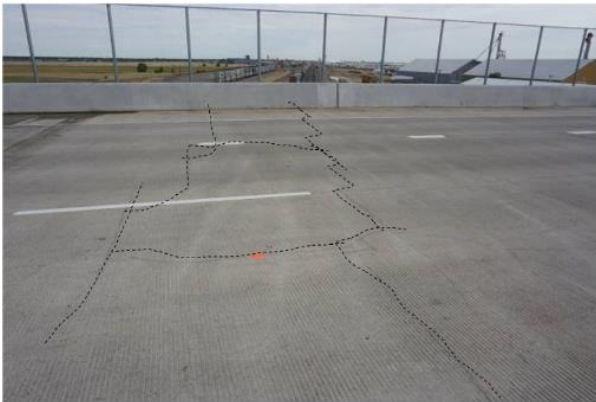
Jump zigzag-type crack propagation on Bridge Deck #1
