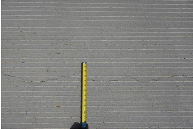
Transverse crack noted at Bridge Deck #1
