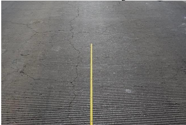
Longitudinal Crack on Bridge Deck #6
