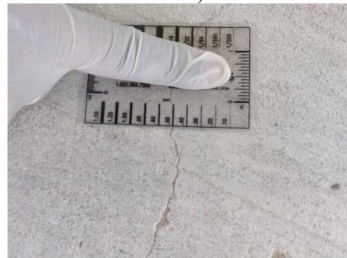
Cracking observed on Span 10 (August 2023)
