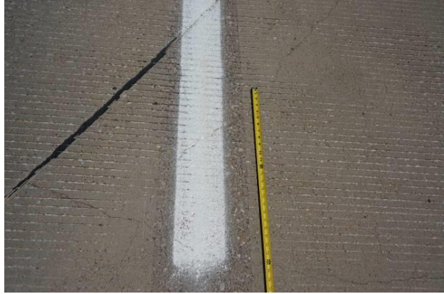
Transverse Crack Propagation on Bridge Deck #7
