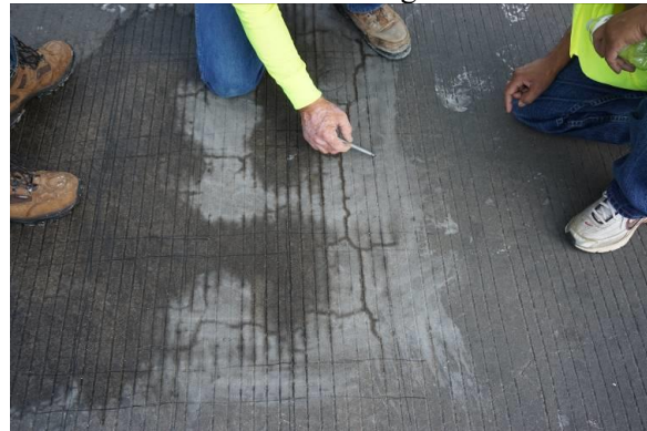
Map crack pattern on Bridge Deck #9
