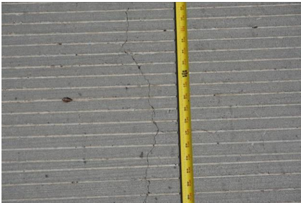
Typ. longitudinal crack propagation on Bridge Deck #4
