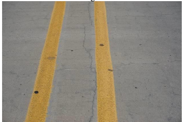
Longitudinal crack propagation for full length along centerline of the Bridge Deck #5
