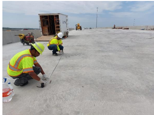
Transverse cracks on deck, Span 5 (August 2023)
