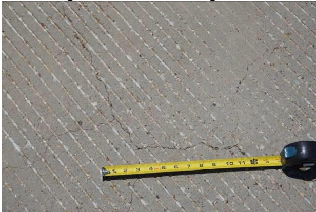
Map Crack Pattern on Bridge Deck #7
