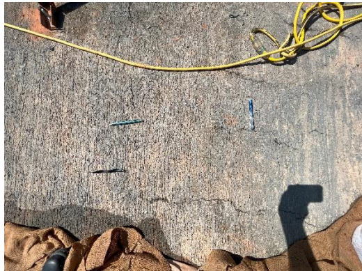
Isolated cracks on deck—FM 2277
