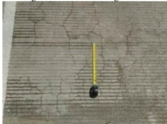
Typical location of map crack pattern on Bridge Deck #2
