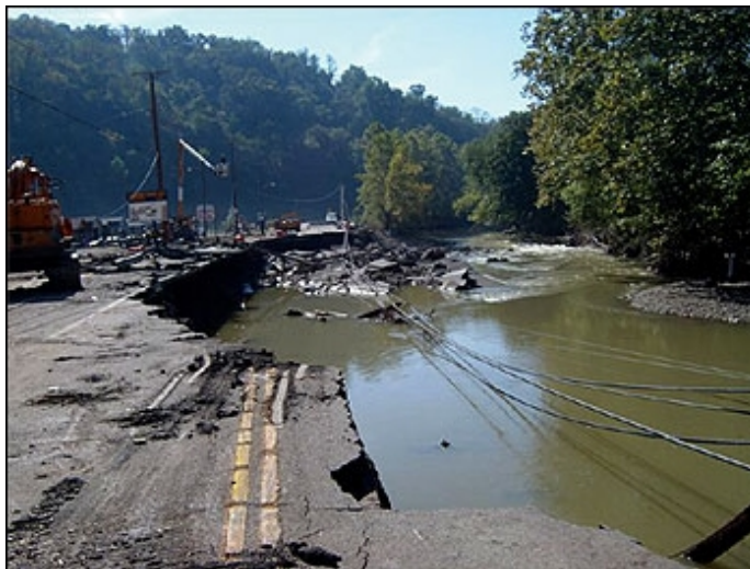
Damaged U.S. 40 washed out from 2004 Flooding near Lansing.
