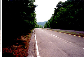
Although closed since 1968, this stretch of pavement between tunnels is in good condition.
