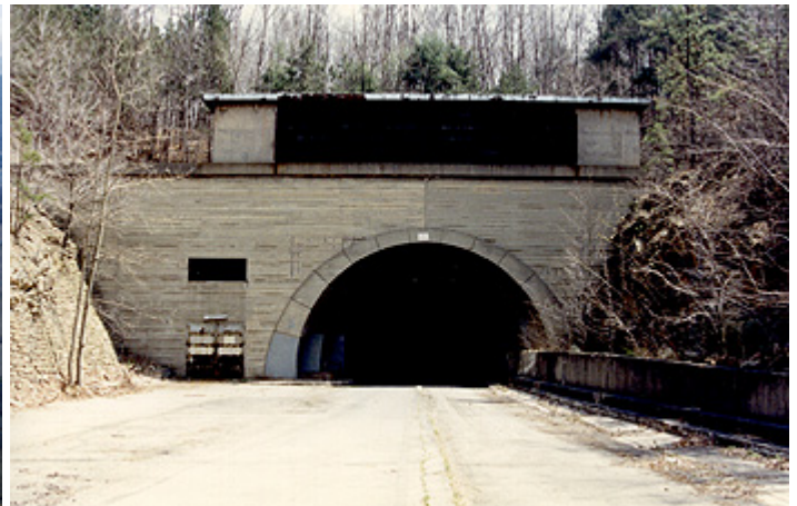
West portal of the Sideling Hill Tunnel. Note the snow removal so that the area could be used.
