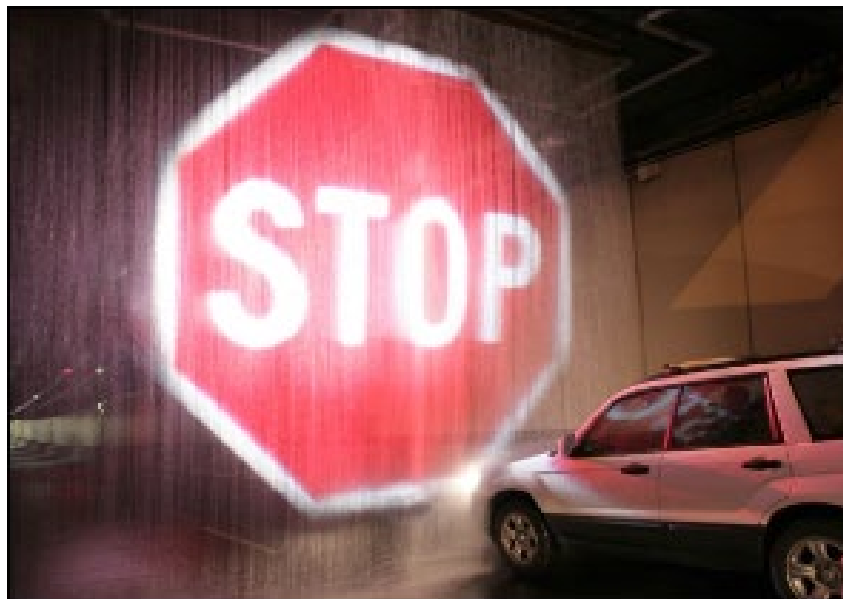
Figure 15. Photo. Softstop™ Barrier System Active Systems installed in the Sydney Harbor Tunnel.
