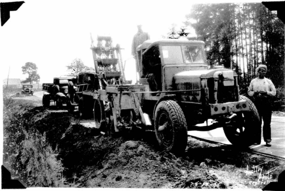
Loader developed by Washington Department of Highways, Maintenance Division. Note teeth mounted ahead of buckets for cutting sod and raking clods into buckets. Truck is towed behind loader while in operation.
