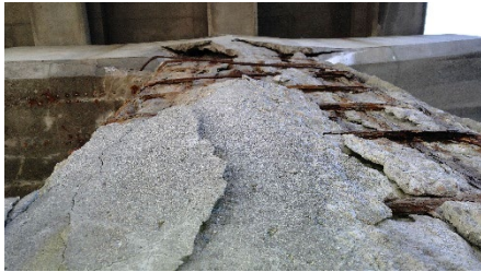
Figure 3 - Severe Delamination / Incipient Spall
