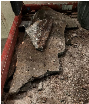
Figure 2 - Removed Concrete from above Highway
