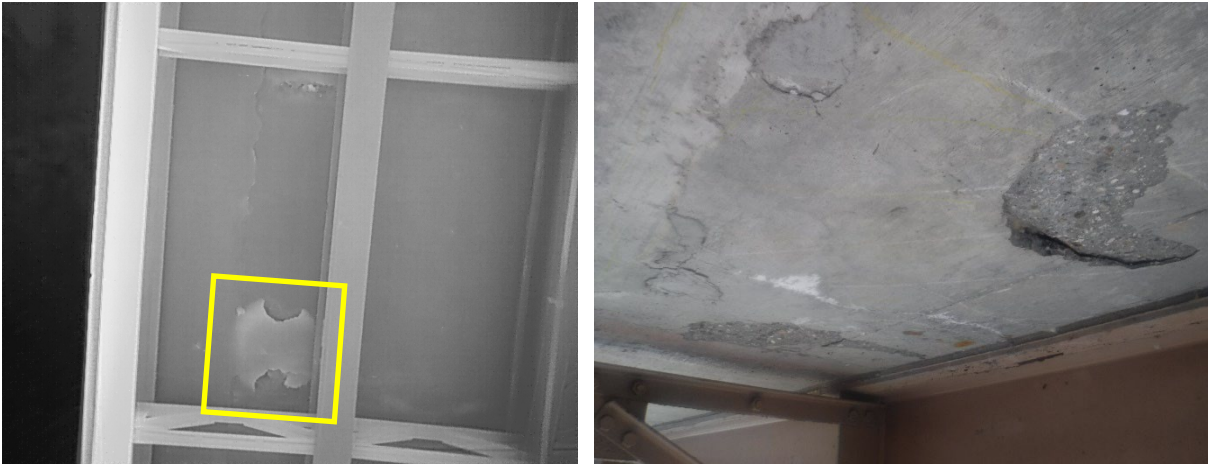
Figure 15 - Delamination without Visible Separation
