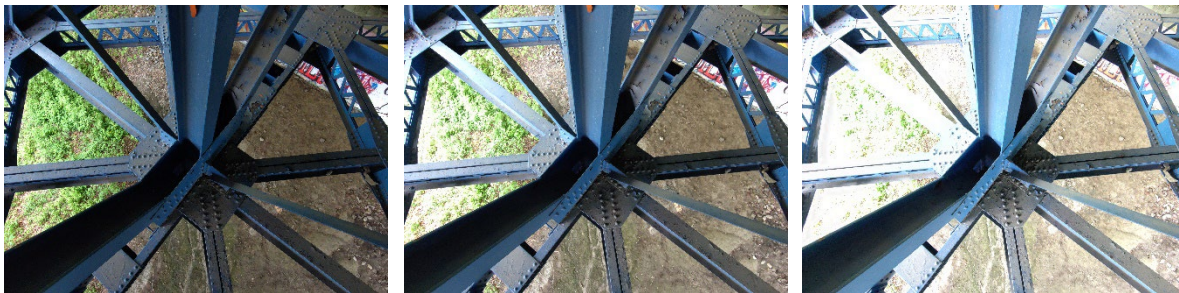
Figure 57 - Inadequate Visual Imagery due to Bridge Geometry and Lighting
