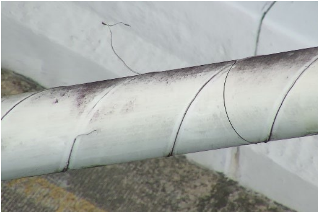
Figure 52 - Helical Bead Damage to Cable Stay
