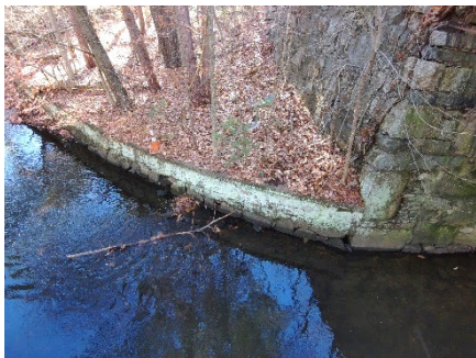
Figure 55 - Channel Wall Deterioration Downstream of Bridge
