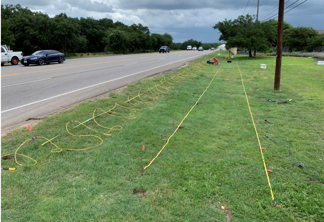
Figure 4.6: Testing on ERT line A, while ERT lines B and C are in preparation.
