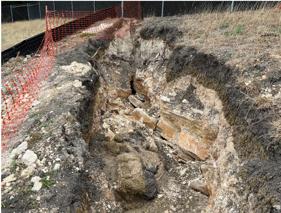
Figure 4.40: Surface opening in the west side of the Southwest Parkway site.
