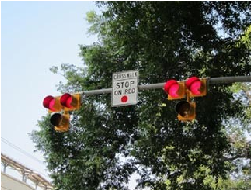
Figure 1.2 – Example PHB Installation
