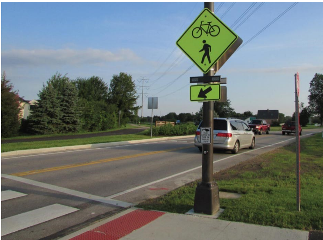
Figure 1.1 – Typical RRFB Installation
