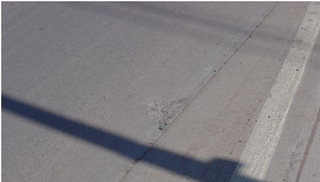
Figure 1.4 Photo. Delamination cracking on US 2 in Wisconsin.
