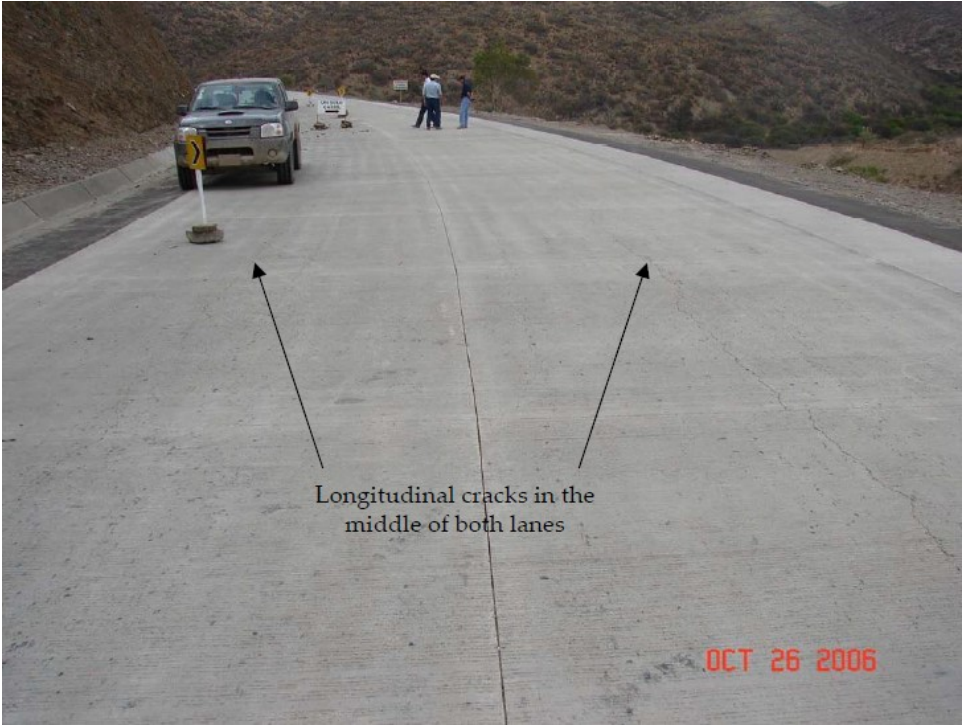
Figure 4.14 Photo. Cracking pattern when both lanes were placed together.
