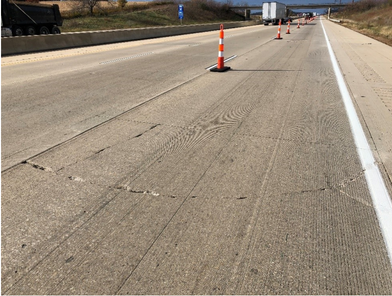
Figure 7.6 Photo. A meandering transverse crack with a partial length longitudinal crack observed on I-39 NB in Columbia County, Wisconsin.
