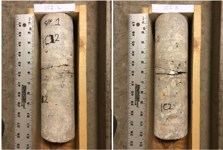
Figure 10.5 Photo. Leave side of 1C2 core (left) and approach side of 1C2 core (right) from I-39 NB in Dane County, Wisconsin.
