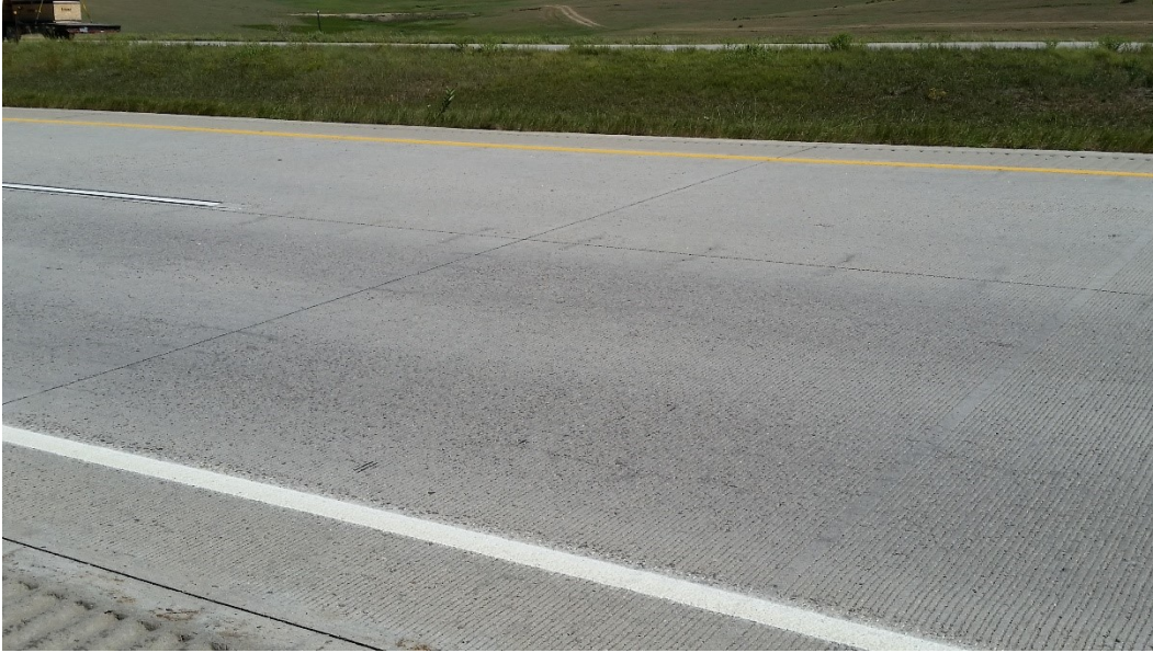
Figure 1.1 Photo. Cracking propagating from both tie bars and dowel bars on I-70 in Colorado.
