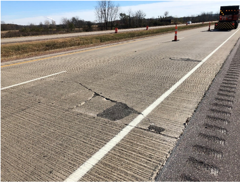
Figure 7.13 Photo. Transverse crack near joint along with associated multiple partial longitudinal cracks and spalling (some filled with asphalt) observed on I-39 SB in Columbia County, Wisconsin.
