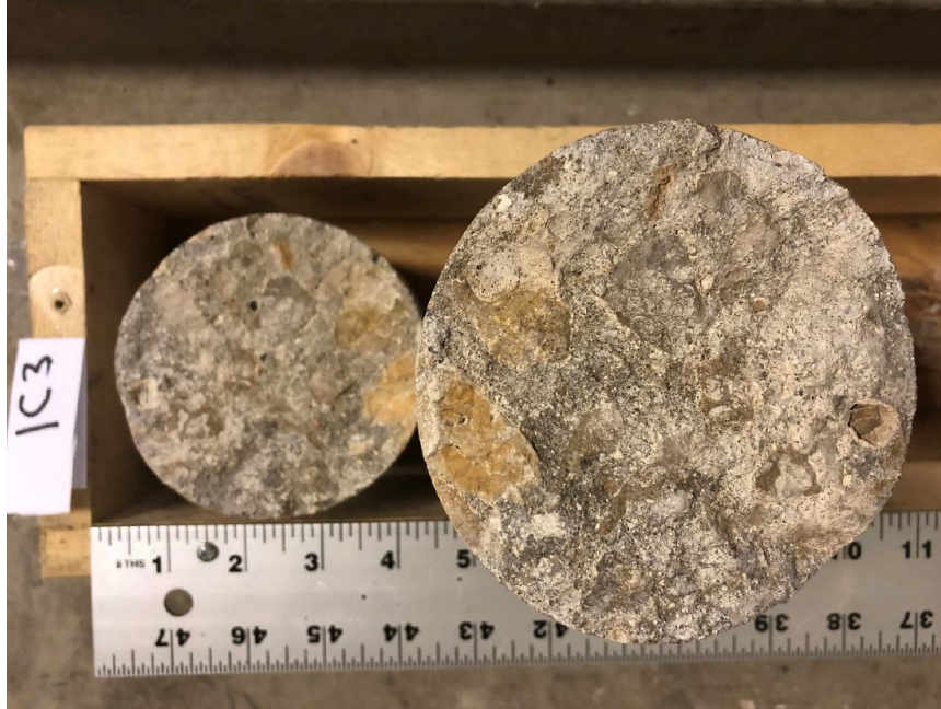
Figure 10.9 Photo. Cross section of 1C3 core from I-39 NB in Dane County, Wisconsin.
