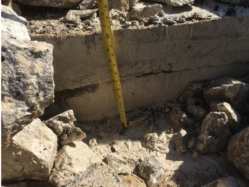
Figure 13.4 Photo. Trench showing delamination cracked concrete from I-39 NB in Dane County, Wisconsin.
