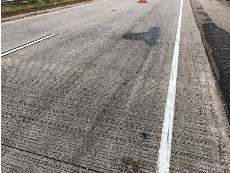
Figure 7.20 Photo. Joint spalling with asphalt patch along with longitudinal crack on US 53 in Eau Claire County, WI.
