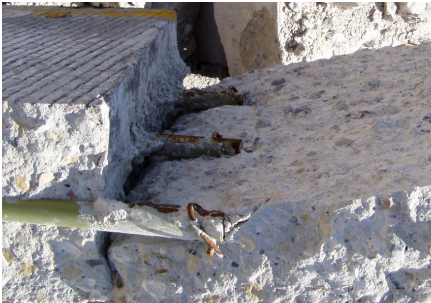
Figure 4.1 Photo. Corner crack showing delamination at dowel depth level and the difference conditions of dowel bars (Rasmussen et al. 2007).
