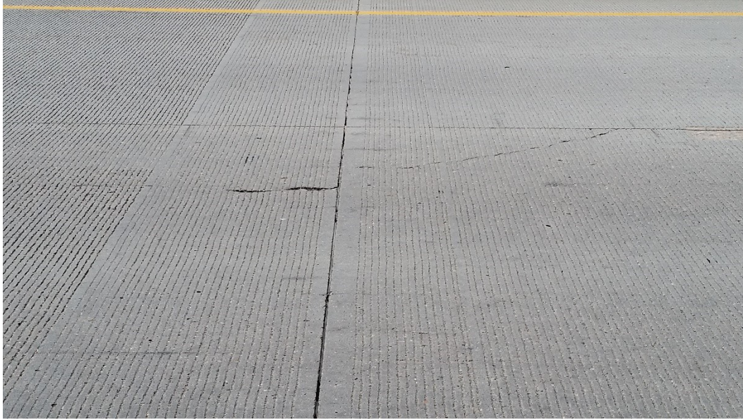
Figure 1.3 Photo. Fully formed longitudinal crack and corner break that initiated as a dowel bar crack on I-70 in Colorado.
