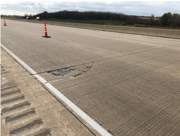
Figure 7.3 Photo. Large corner break partially patched with asphalt observed on I-39 NB in Dane County, Wisconsin.
