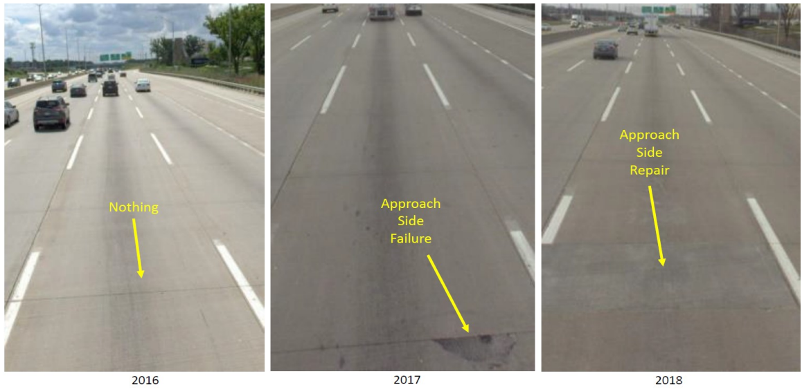
Figure 8.5 Photo. Spall progression from 2016 through 2018 taken using a front facing camera on I-94 EB, Lane 3, MP 18.55 at the Illinois Tollway.
