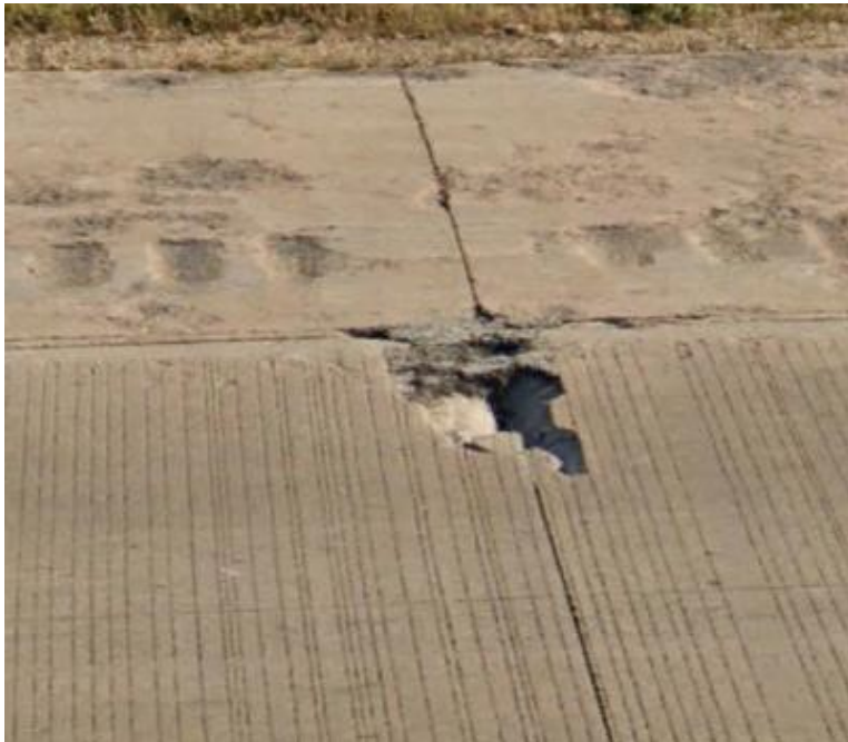
Figure 7.1 Photo. Corner break observed on I-39 NB in Dane County, Wisconsin.
