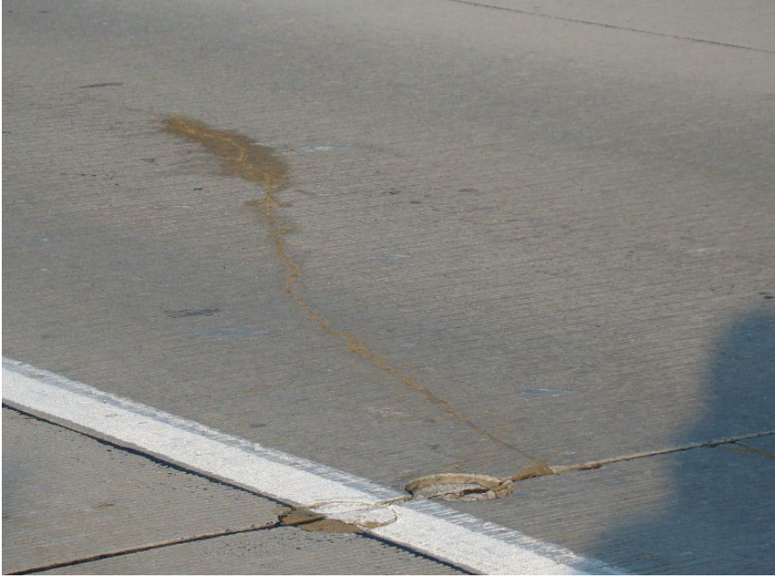
Figure 3.12 Photo. Longitudinal shear restraint crack of dowel initiating over dowels at two locations on opposite sides of the joint (Harrington et al. 2018).
