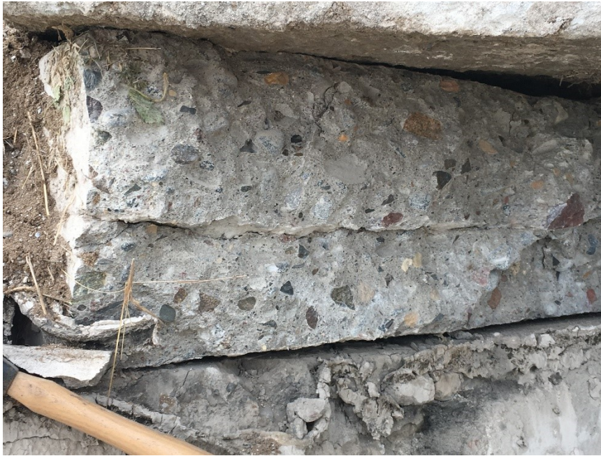
Figure 13.1 Photo. Stacked slabs of trenched concrete at the disposal/recycle yard from TH 610 in Hennepin County, Minnesota showing horizontal crack at about mid slab depth.
