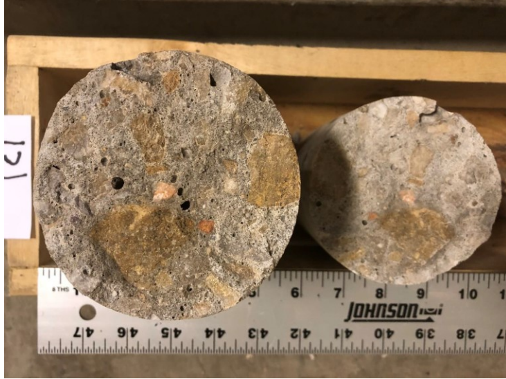
Figure 10.3 Photo. Cross section of 1C1 core from I-39 NB in Dane County, Wisconsin.
