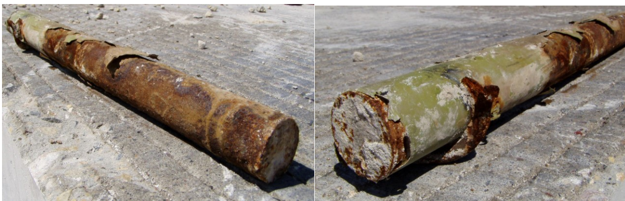
Figure 4.2 Photo. Dowel bar conditions showing ineffectiveness of epoxy coating and abrasion (Rasmussen et al. 2007).
