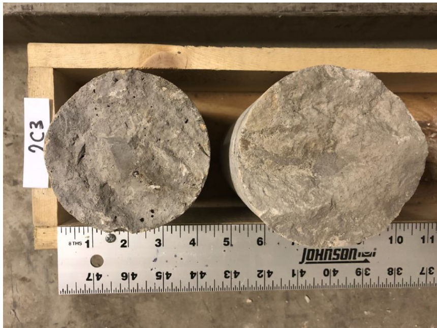
Figure 10.25 Photo. Cross section of 2C3 core from I-39 NB in Dane County, WI.
