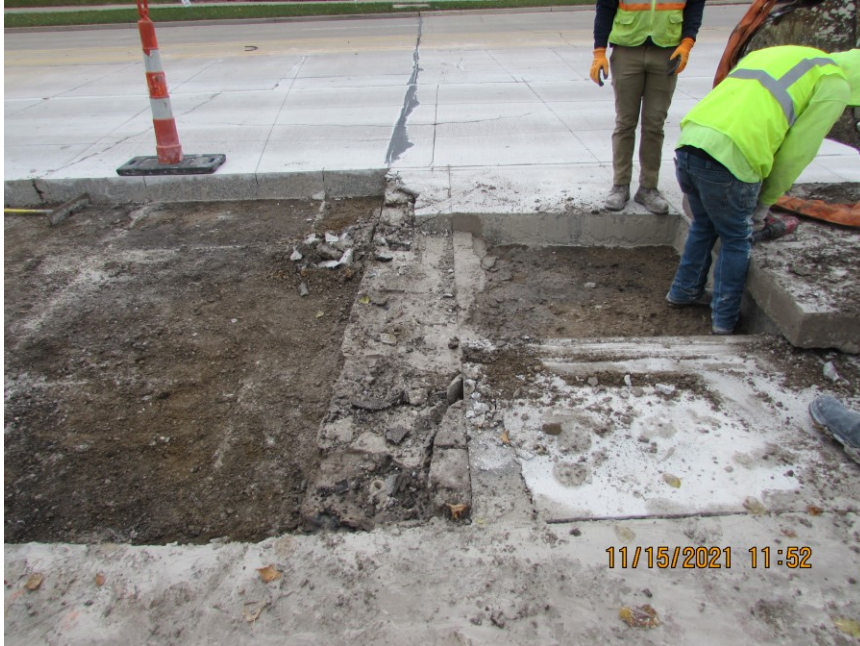
Figure 13.6 Photo. Trench showing concrete split at around mid-depth during trenching from a city street in Central Illinois on a relatively new (less than 3 years) concrete pavement.
