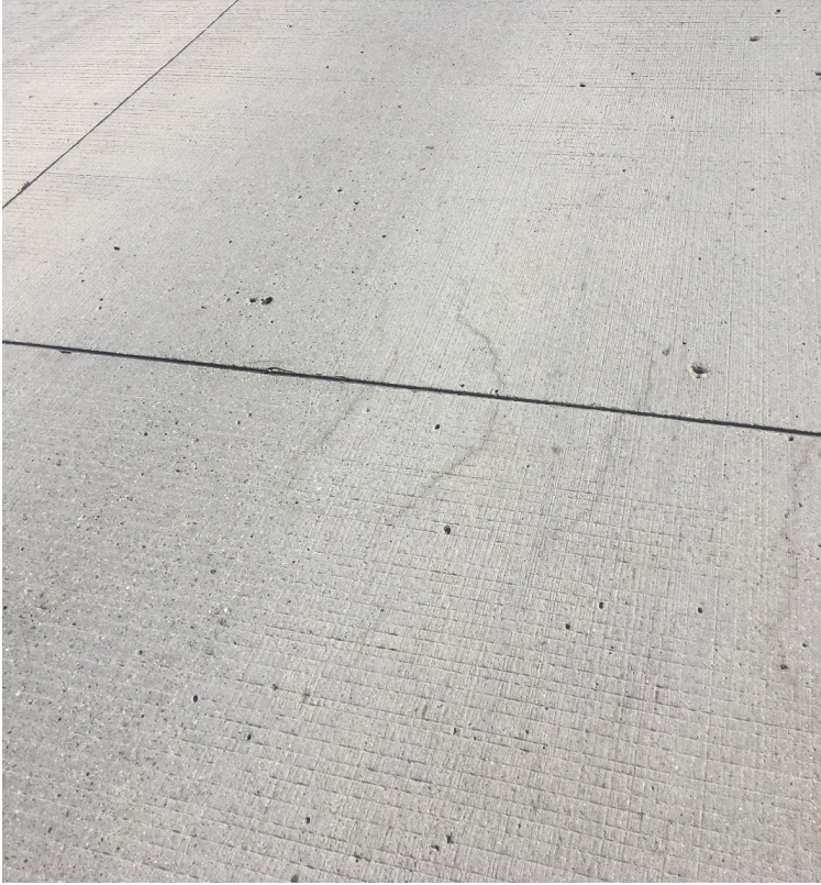
Figure 4.16 Photo. Crack over dowel bars in SPS-2 in North Dakota.
