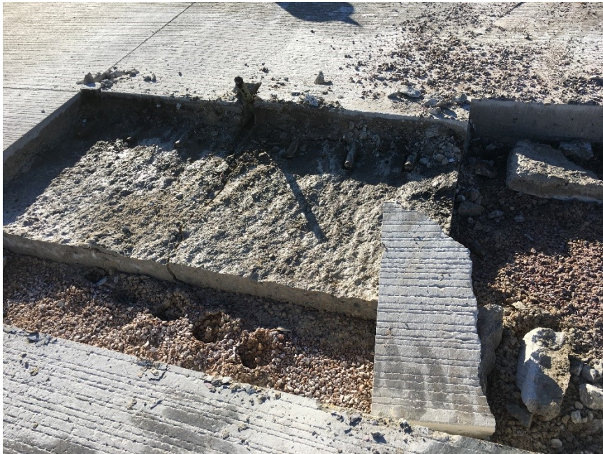
Figure 13.3 Contour Plots. Trench showing delamination cracked concrete from undocumented site in Wisconsin.
