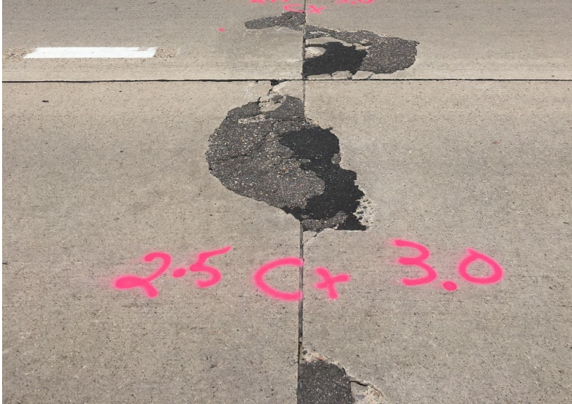
Figure 7.16 Photo. Advanced large joint spalls with asphalt patches on TH 610 in Hennepin County, MN.
