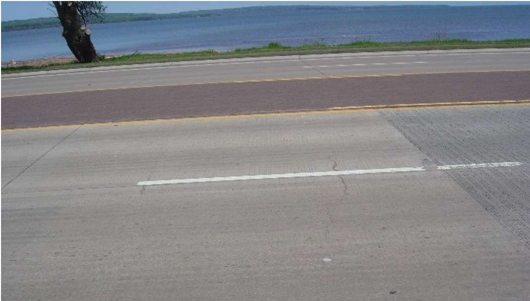
Figure 1.2 Photo. Cracking propagating from tie bars on US 2 in Wisconsin.
