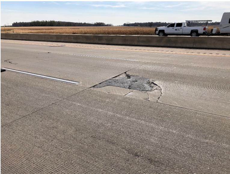
Figure 7.5 Photo. A large spall partially filled with asphalt observed on I-39 NB in Columbia County, Wisconsin.
