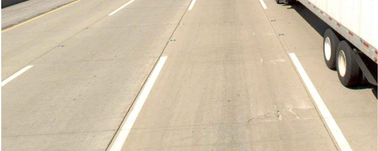
Figure 7.14 Photo. Early stage joint deterioration on I-94 at the Illinois Tollway.
