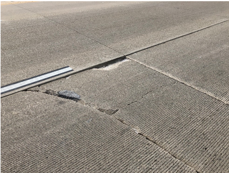
Figure 7.7 Photo. Full length transverse crack with a partial length longitudinal crack observed on I-39 NB in Columbia County, Wisconsin.
