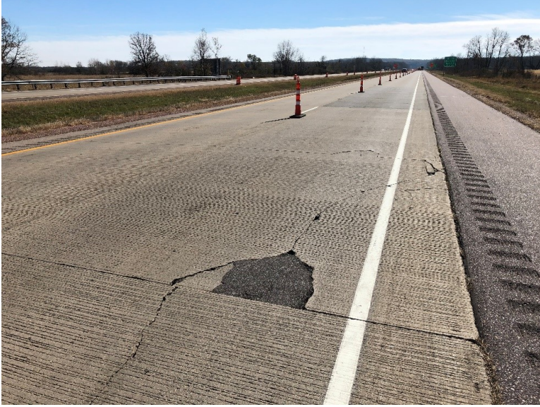
Figure 7.10 Photo. Large spall partially filled with asphalt along with meandering longitudinal crack observed on I-39 SB in Columbia County, Wisconsin.
