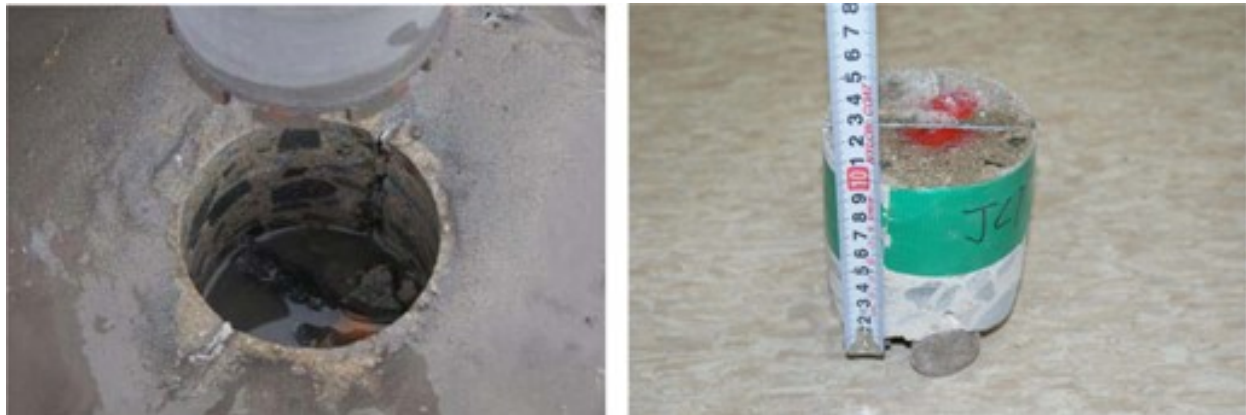
Figure 4.5 Photo. Core taken from longitudinal crack location (Seo and Kim 2012).
