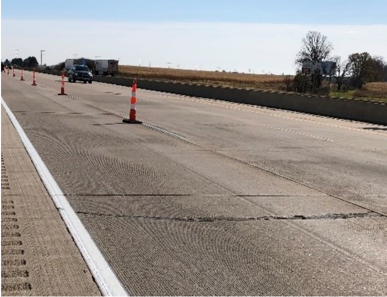
Figure 7.4 Photo. Full length transverse crack about two to three feet from transverse joint observed on I-39 NB in Dane County, Wisconsin.
