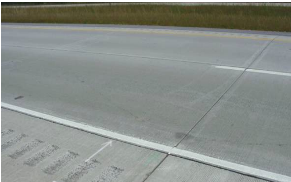
Figure 4.11 Photo. Characteristic pattern of edge-restraint cracking.
