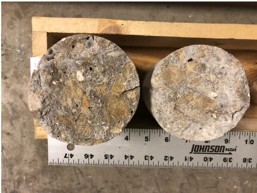
Figure 10.13 Photo. Cross section of 1C5 core from I-39 NB in Dane County, Wisconsin.
