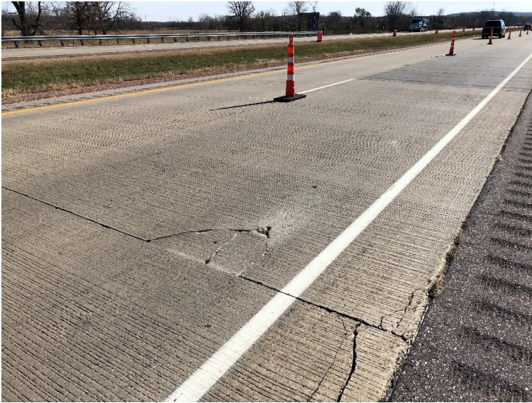
Figure 7.11 Photo. Large unrepaired spall observed on I-39 SB in Columbia County, Wisconsin.
