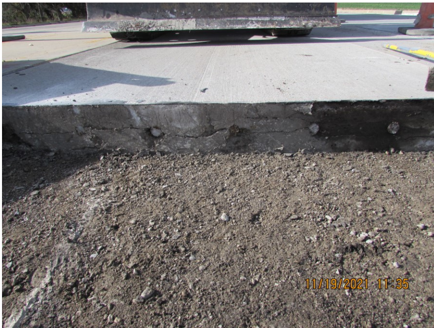
Figure 13.5 Photo. Trench showing delamination cracked concrete from a city street in Central Illinois on a relatively new (less than 3 years) concrete pavement.
