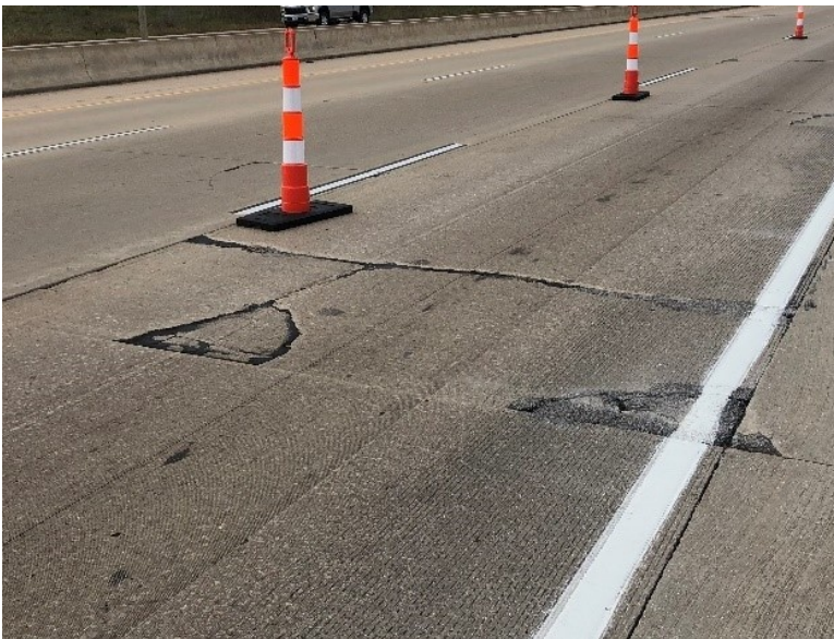
Figure 7.9 Photo. Full length transverse crack with a partial length longitudinal crack and compound spalls observed on I-39 NB in Columbia County, Wisconsin.
