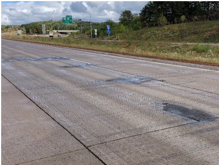
Figure 7.21 Photo. Several consecutive joints with spalling filled with asphalt patches on US 53 in Eau Claire County, WI.
