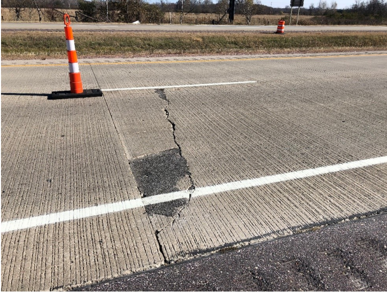
Figure 7.12 Photo. Large spall partially filled with asphalt along with meandering transverse crack observed on I-39 SB in Columbia County, Wisconsin.
