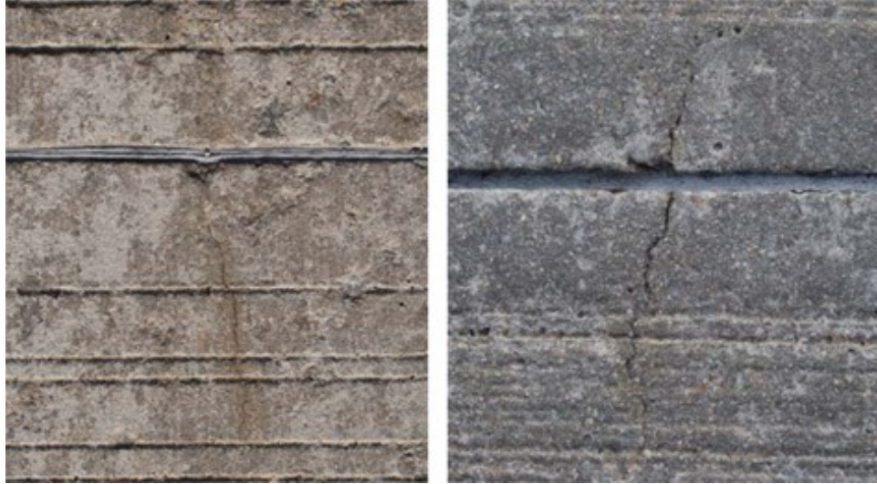
Figure 4.4 Photo. Longitudinal cracks at joint (Seo and Kim 2012).
