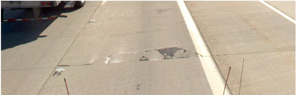
Figure 7.15 Photo. Advanced joint deterioration with patching material on I-94 at the Illinois Tollway.
