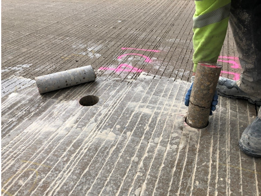
Figure 10.12 Photo. Two cores on I-39 NB in Dane County, Wisconsin, with no distresses observed at the surface. One core away from the joint is intact whereas the core closer to the joint had delamination cracking.
