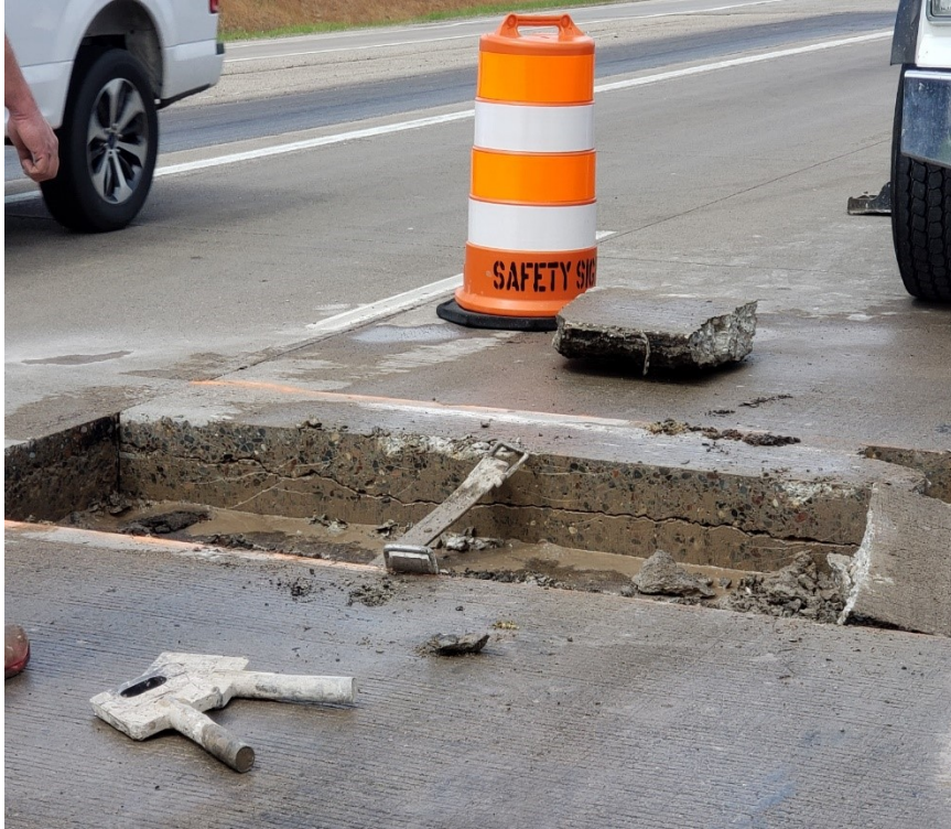
Figure 13.2 Photo. Trench showing delamination cracked concrete from TH 610 in Hennepin County, Minnesota.
