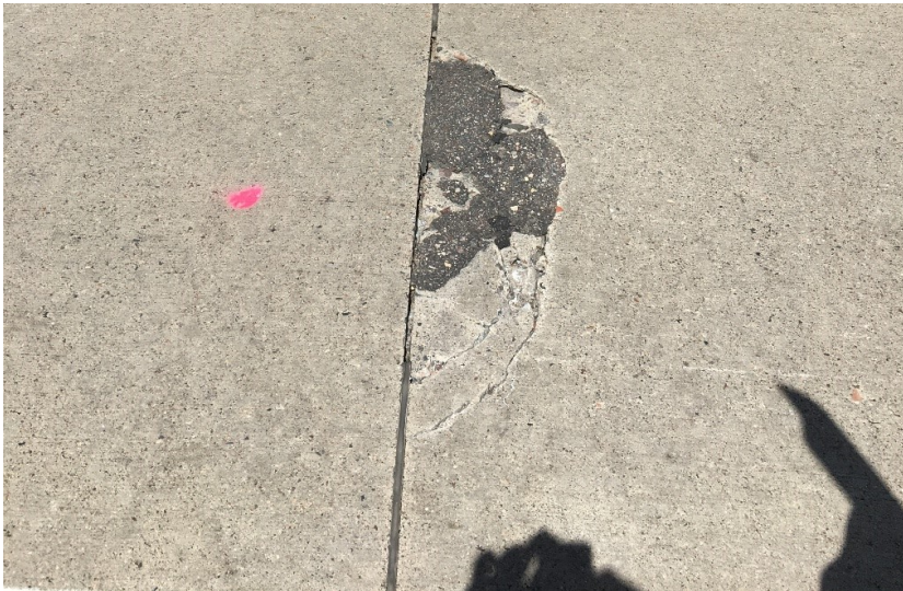
Figure 7.17 Photo. Joint deterioration with asphalt patch on TH 610 in Hennepin County, MN.
