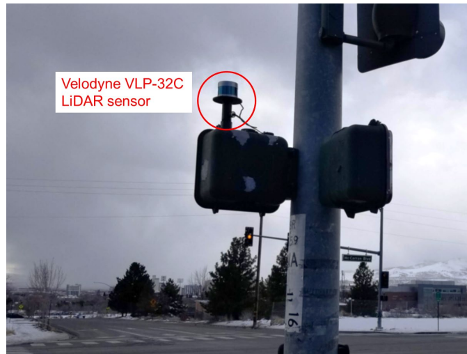
Figure 2-5. A LiDAR sensor installed on a traffic signal lighting pole at a road intersection.
