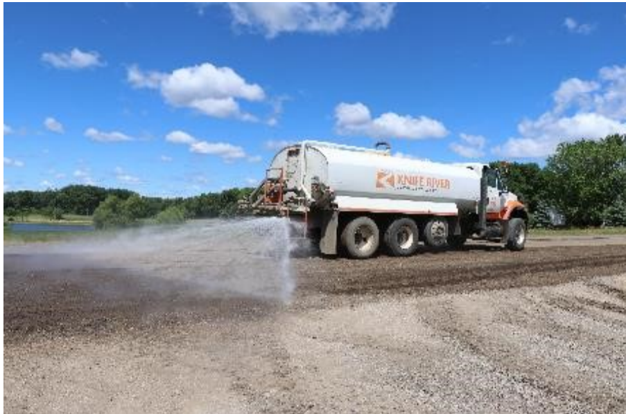
Figure 43. Spraying water from the storage tank to moisten FDR materials before milling
