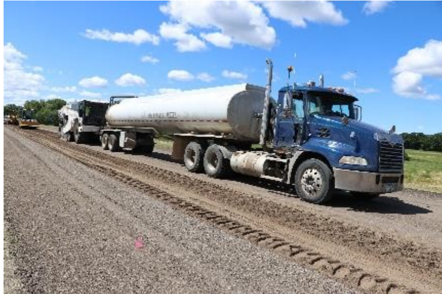
Figure 44. Applying chemical stabilizer and mixing with RAP material by using a reclaimer
