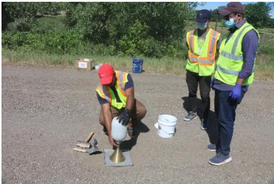
Figure 49. Measuring the in-place density of stabilized FDR base by using sand cone apparatus
