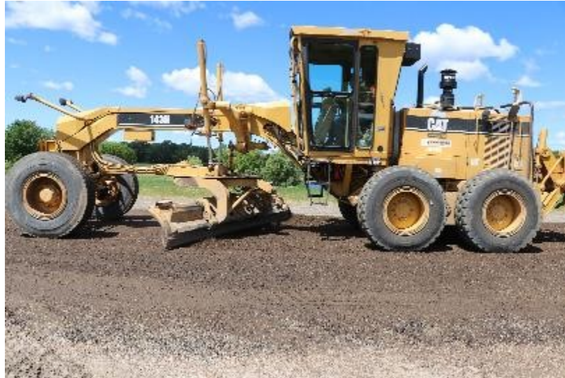
Figure 46. Blading and leveling the surface of the treated RAP base layer by using a motor grader
