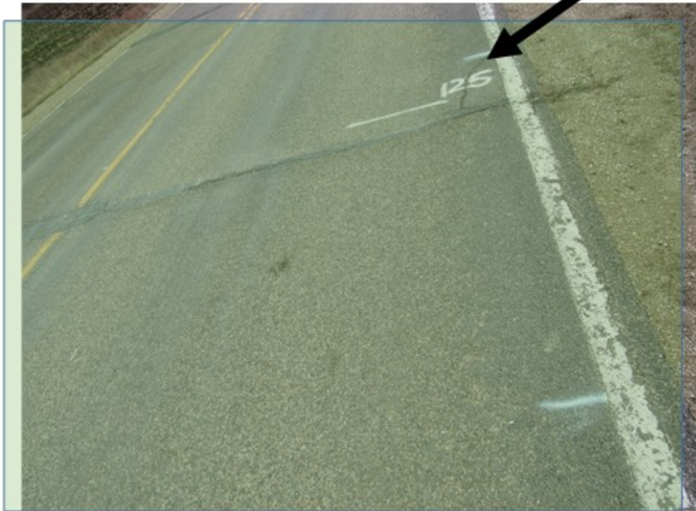
Figure 3.15 Secondary Cracking, Section 1B
