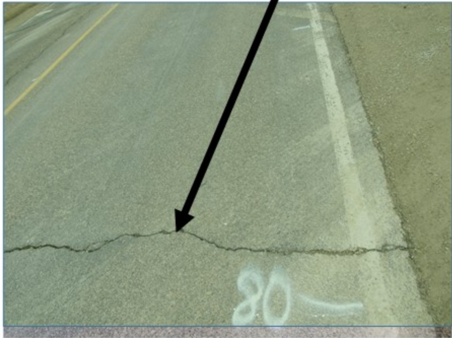
Figure 3.14 Transverse Crack in Section 1B
