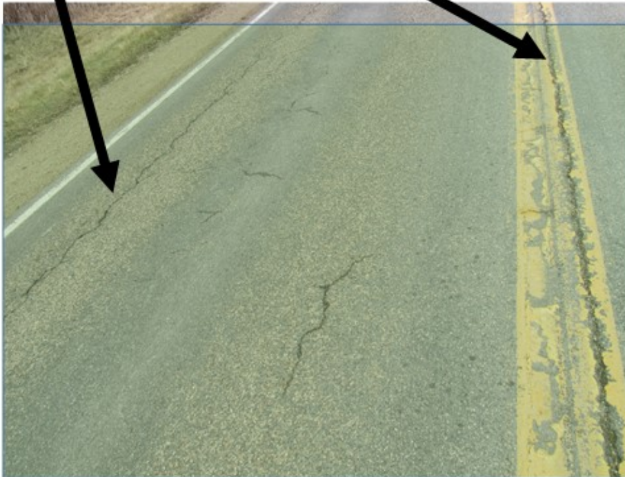
Figure 3.11 Wheel path Cracking Observed in Section 1A
