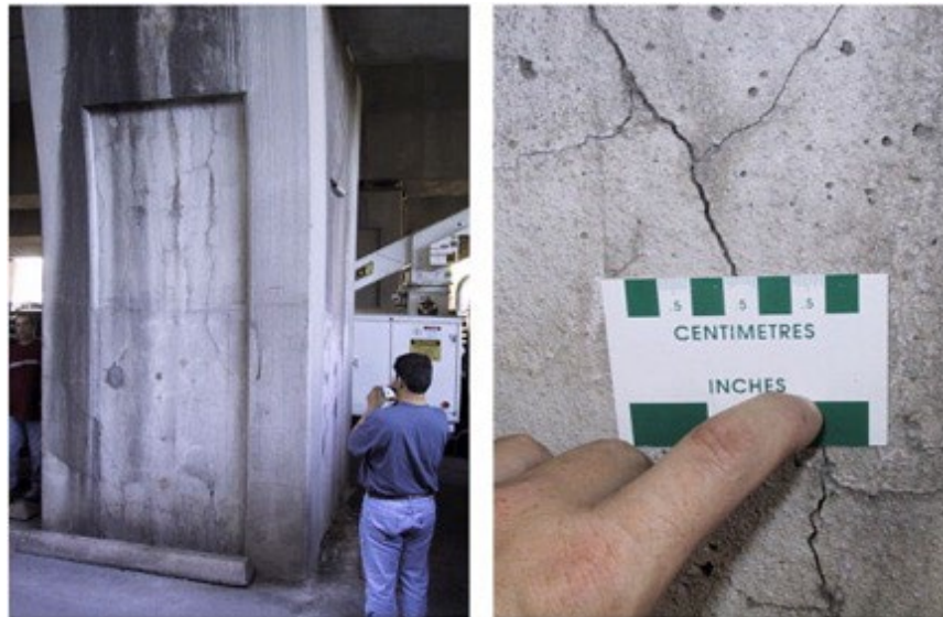
Figure 11.5: Concrete Structures Affected by DEF. [12]
