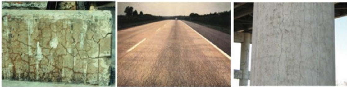
Figure 11.4: Concrete Structures Affected by ASR [2]
