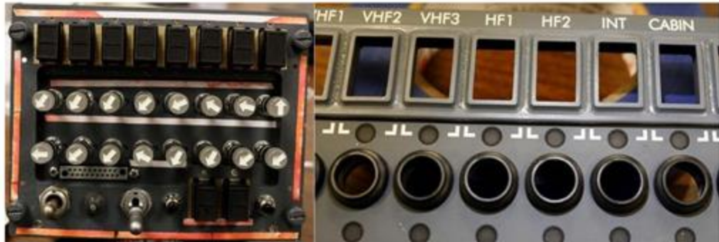
Figure 22: Indications of ingress in [redacted] ACP under the light plate and residue between button cutouts
