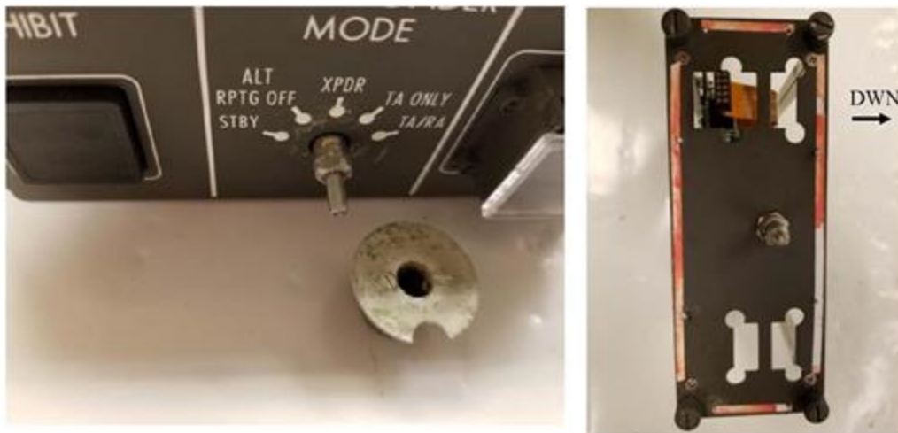
Figure 58. The [REDACTED] Alerting and Transponder Control had significant fluid ingress behind the light plate. Corrosion between the selector knob set screw and shaft was sufficient to preclude hand disassembly. Residue was present between the knob and face plate.
