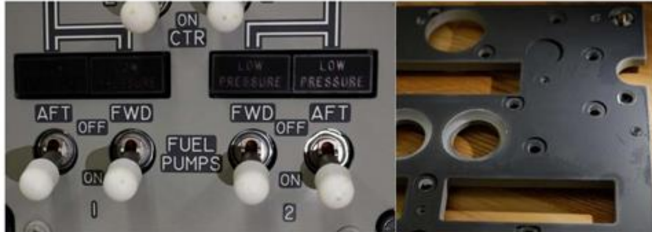
Figure 17: Calla 1452 residue on white switches and moisture on back side of light plate of fuel control panel
