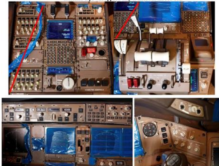
Figure 2: LRUs subjected to e-spray (LRUs under red line were not e-sprayed)
