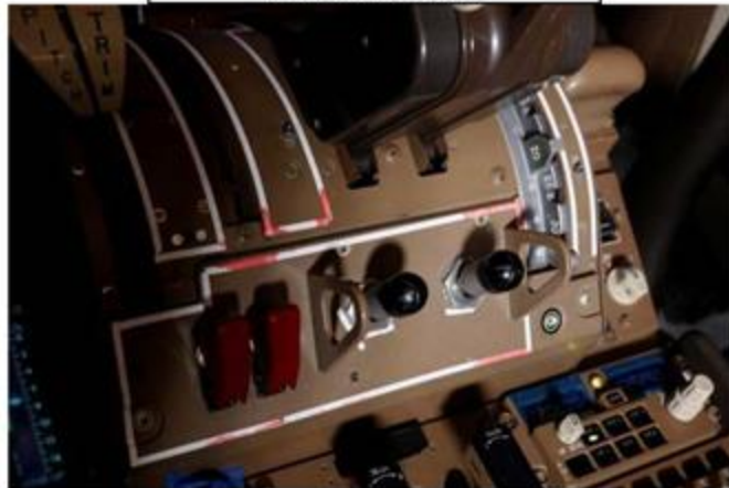
Figure 3: Largest amount of liquid ingress (indicated by red spots) under the light plates of the control stand assembly
