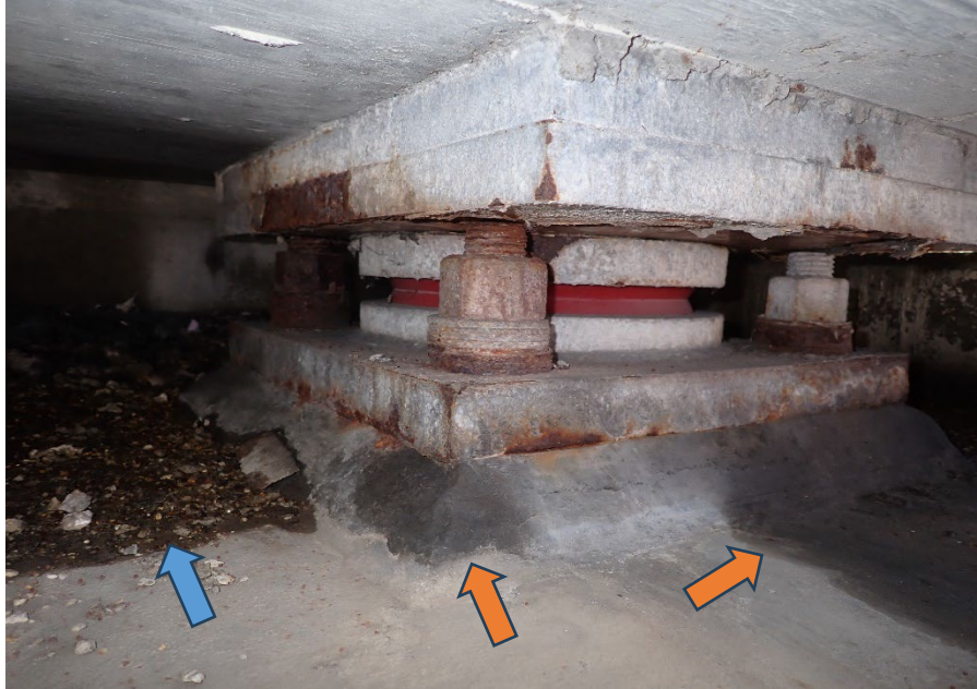
Figure 56. Photo of a pot bearing below a bridge joint with moist concrete that identifies water infiltration occurred (orange arrows) and debris accumulation (blue arrow). An elastomeric bearing may be placed in a similar environment.
