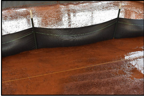
(a) undermining and sagging
