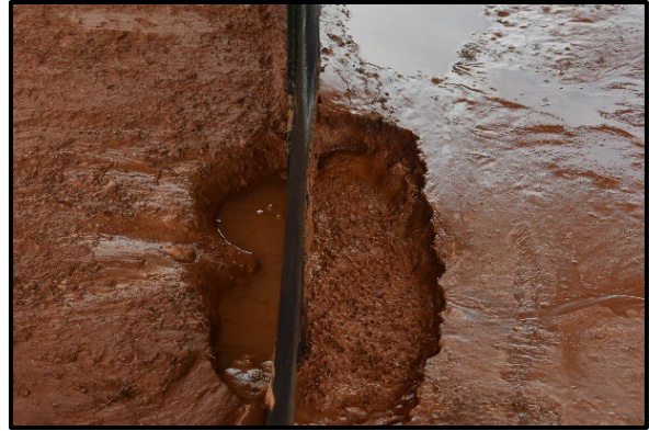
(b) trench failure
