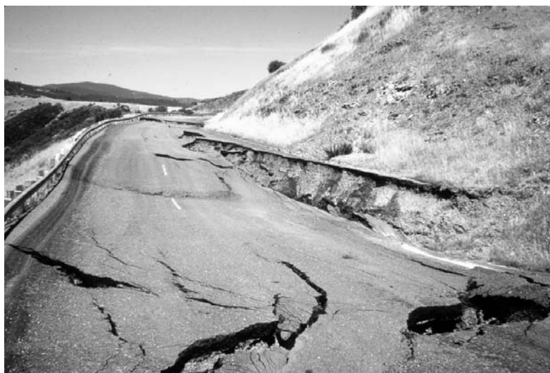
Figure 1-2: Side Hill Fill Settlement
