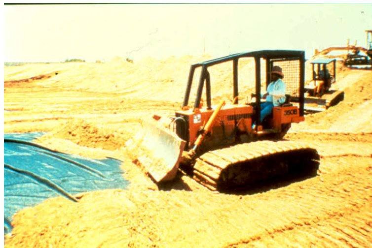
Figure 7-10. Reinforced embankment construction; a) geosynthetic placement; b) fill dumping; and c) fill spreading.
