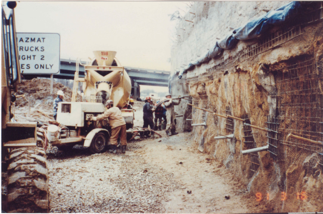
Figure 18. Construction of Soil Nailed Retaining Wall under GWMP Bridge Abutment Prior to Shotcreting.
