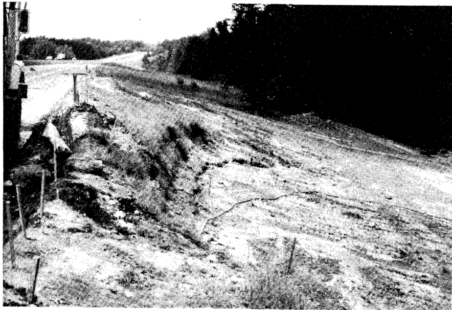
Photo 10 Same scarp, different view and after additional slurry was injected.
