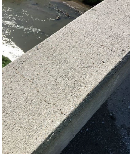
Figure 1.2 Early-age shrinkage cracks in bridge rails
