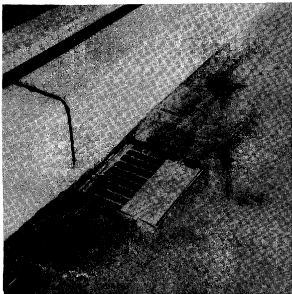
Fig. 1 Grand Ave OH (Br 24-288R/L) Test Drain - hand packed from top with damp debris.
