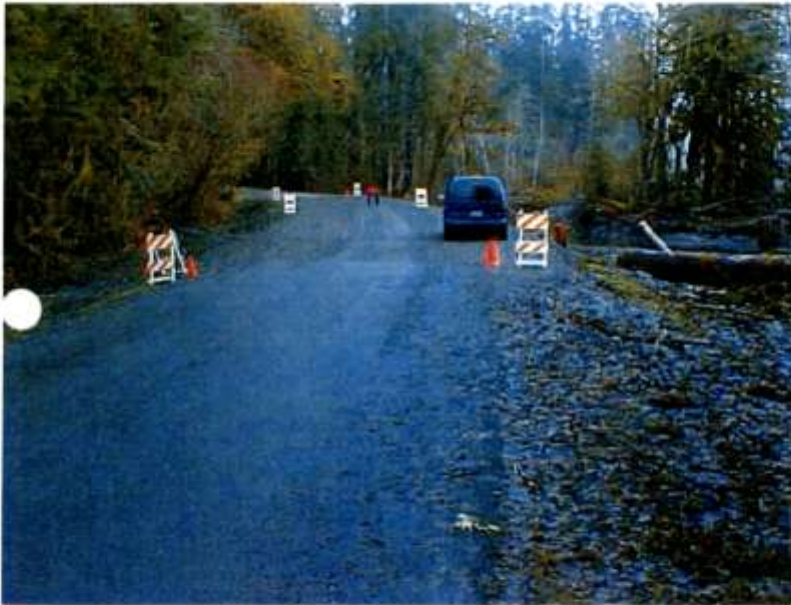
Roadway Washout - emergency/permanent repairs completed (without final surfacing and log crib mitigation)
