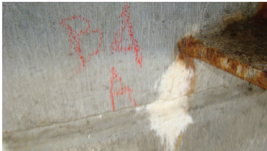
Figure 56. Bridge 07335, Bent 4, Girder 4, Efflorescence Close-up
