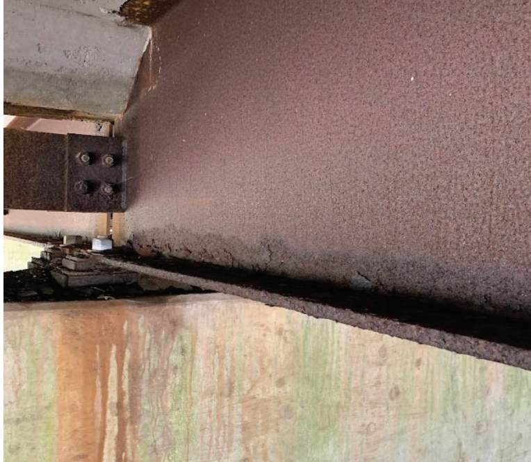
Figure 47. Bridge 06319: CS 3 and CS 4 on Interior Girder
