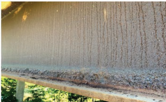
(c) ARDOT Bridge B6507 with an 1/8" pit: CS 3
