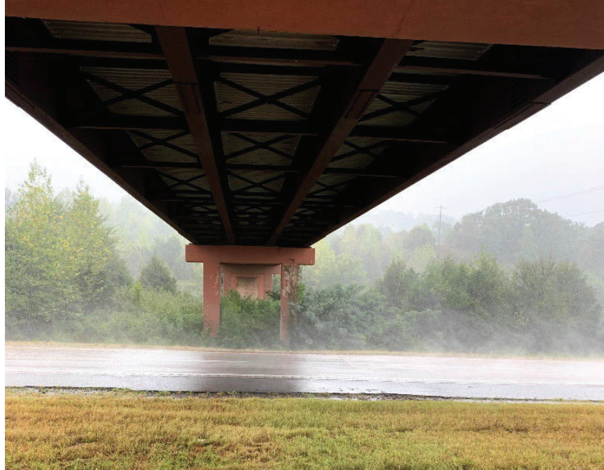
Figure 25. Overpass Where Vehicular Traffic Safety Management is Warranted
