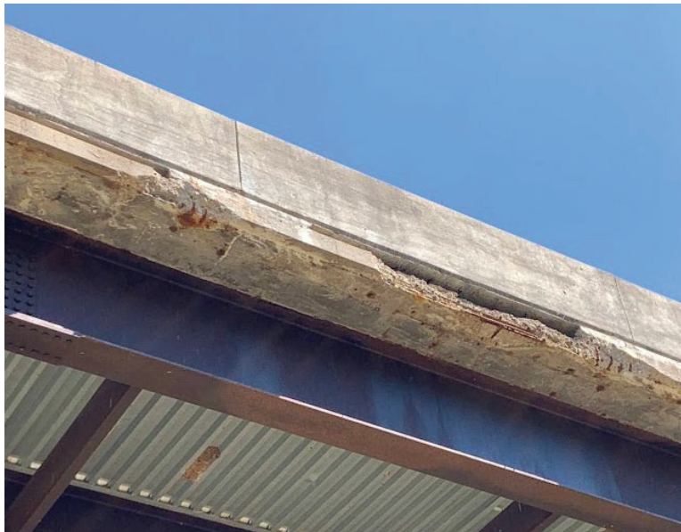
Figure 45. Bridge 06371: CS 2 and CS 3 on Web
