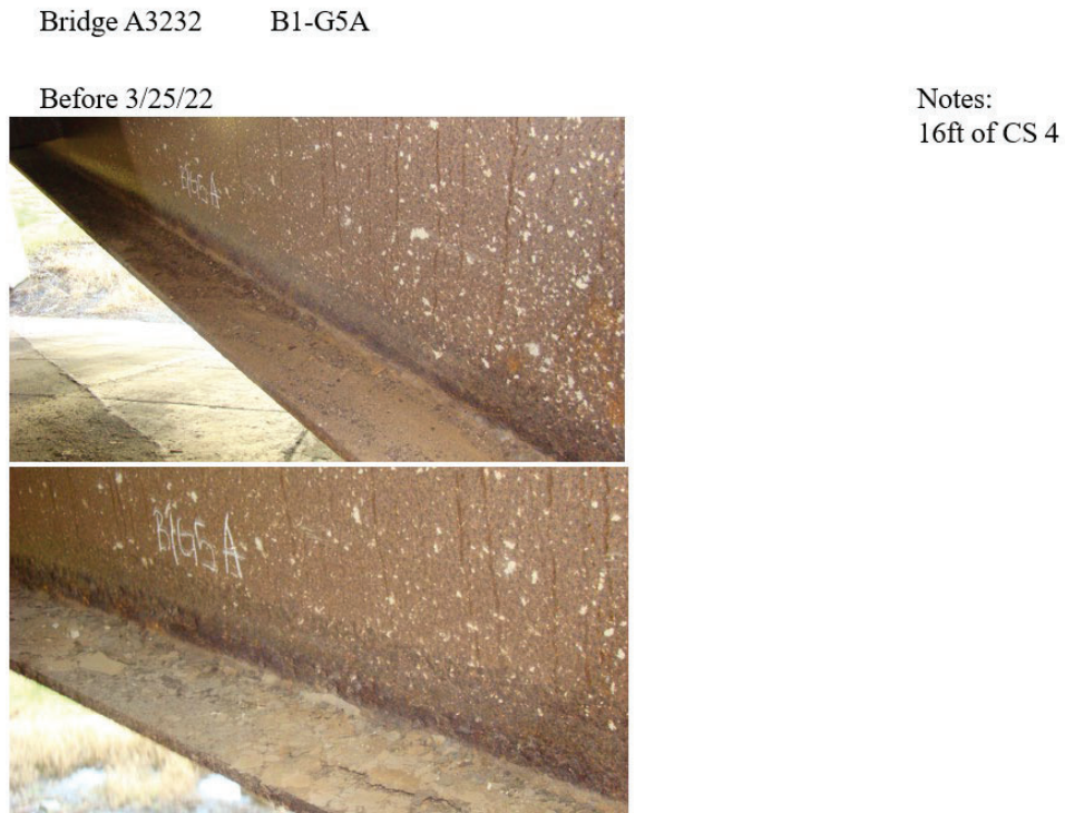
Figure 37. Before and After Cleaning Rust Flakes
