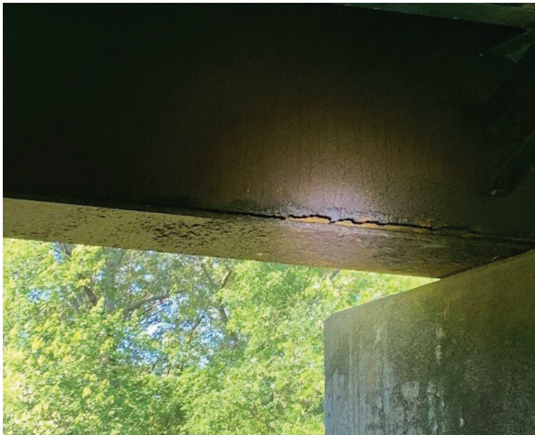
Figure 48. Bridge 06319: CS 3 and CS 4 near End Abutment
