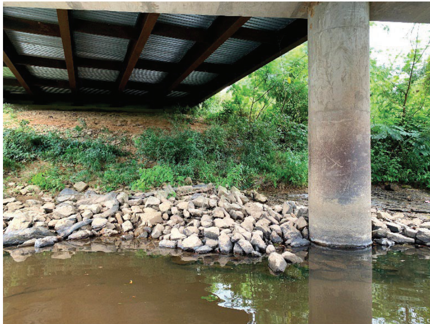
Figure 26. Exposed Fabric Bed near Pier Columns
