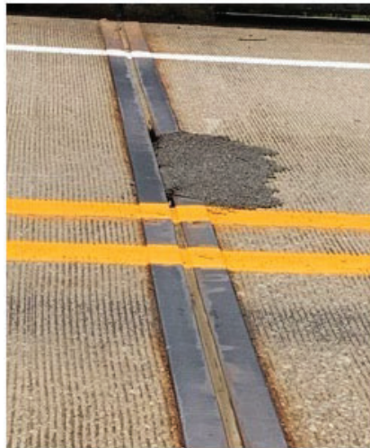
(c) Asphalt Damage
