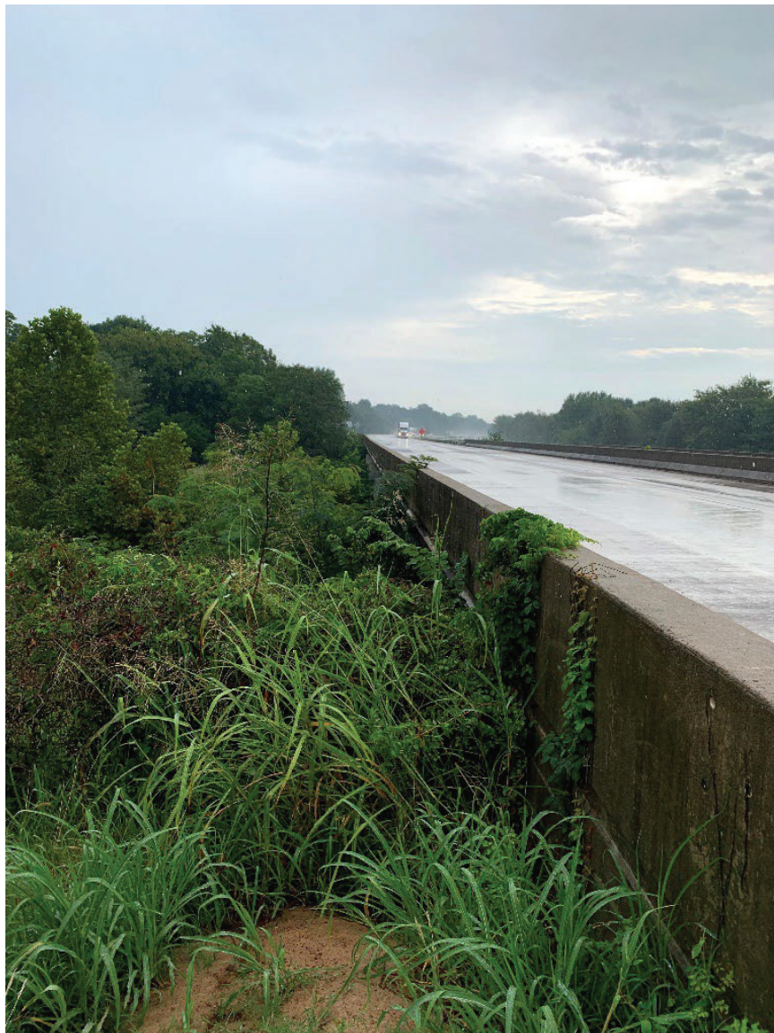
Figure 19. Bridge A6820 Enclosed with Vegetation
