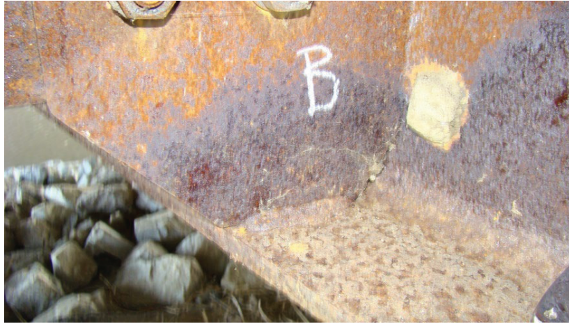
Figure 57. Bridge 07335, Bent 4, Girder 4, Corrosion at Diaphragm Connection
