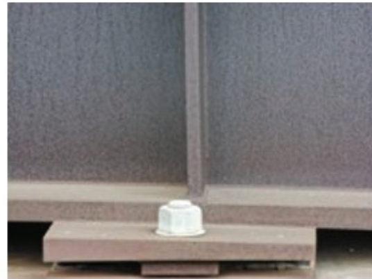
(b) Close-up of girder bearing at bridge pier cap using zoom from UA location in (a)
