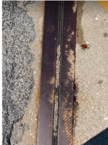
(a) Asphalt in Joint Sealant
