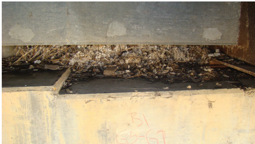
Figure 63. Debris at South Abutment (Bent 1)
