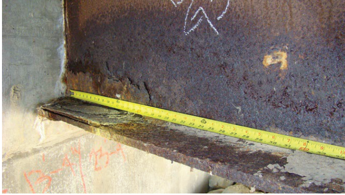
(a) Efflorescence at Girder-Abutment
