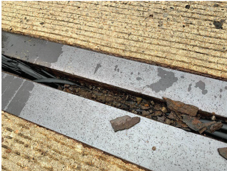
Figure 22. Corrosion and Debris Collected in the Expansion Joint
