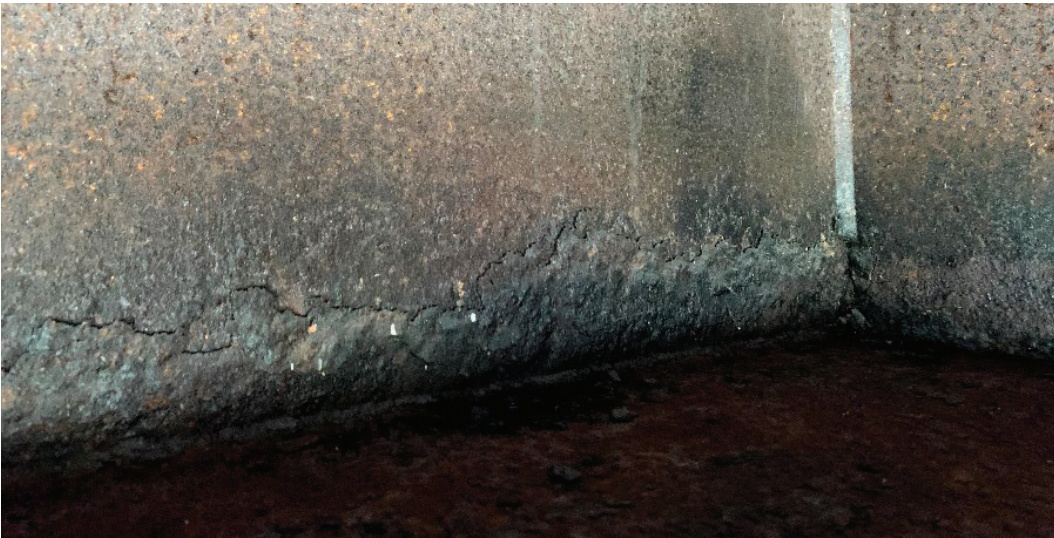
Figure 14. Rust with Rust Inhibitor
