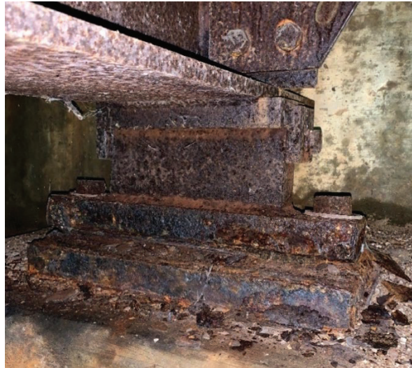
Figure 23. Bearing Corrosion: CS 4
