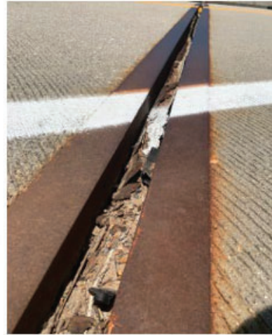
(b) Damaged Sealant and Debris
