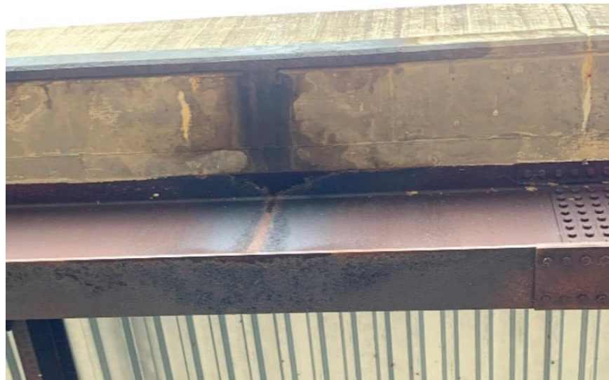
Figure 24. Girder Corrosion due to Improper Deck Drainage
