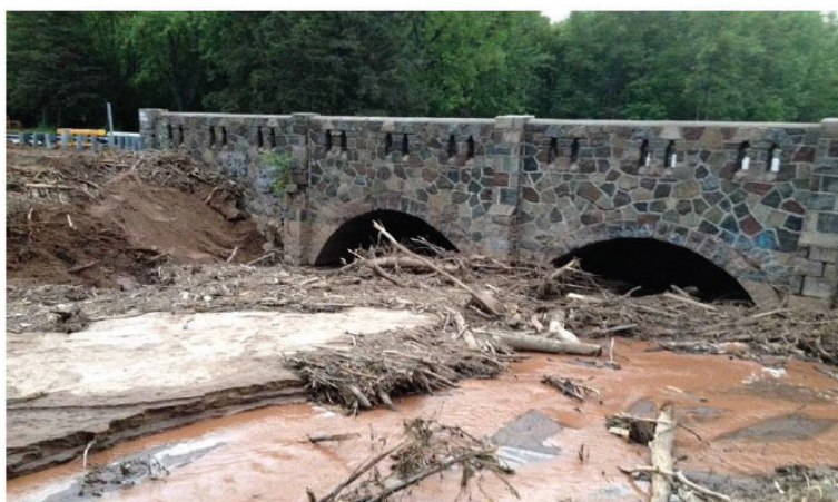
Figure 8. Flooding in MnDOT Obstructing a Historic Bridge (Parsons Brinckerhoff and Catalysis 2014)
