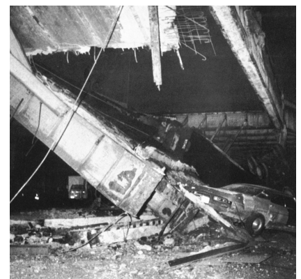
On December 15, 1973, the northbound lanes of the West Side Highway collapsed between Little West 12th Street and
