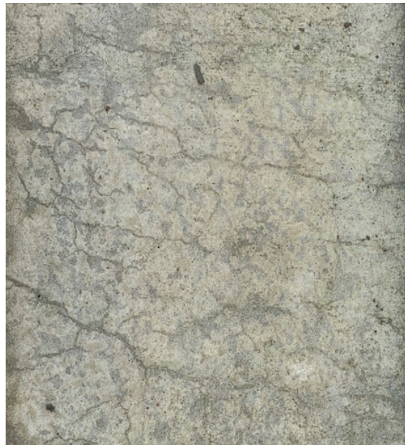
Figure 3. Example of Plastic Shrinkage Cracks in Hardened Concrete
