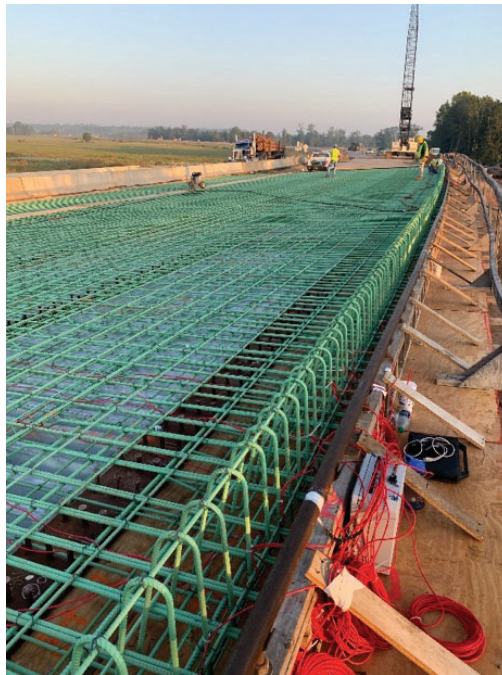
Figure 11. Bridge No. 07364 While Sensors were Being Installed (DAQ box shown in lower right of image)
