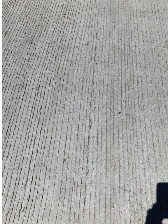
Figure 64. Cracking in No. Bridge 07364 Noticed After Deck Pour (Photo credit Jason Eford)
