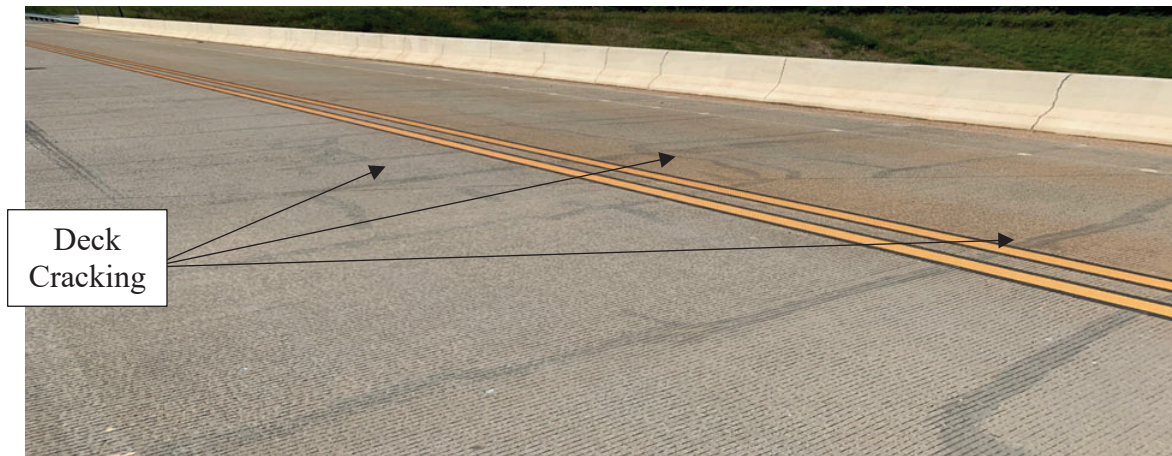
Figure 1. Cracking Prior to Applying Live Loads
