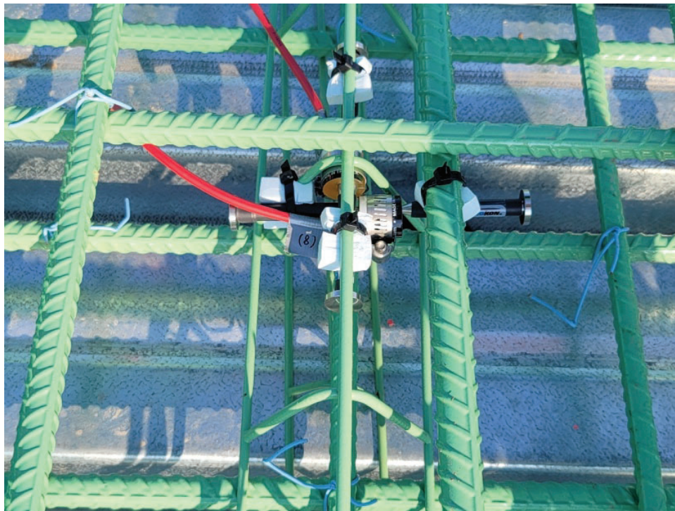
Figure 20. Example of Sensor Installation on Bridge No. 07473, top to Bottom is Longitudinal Direction of Bridge
