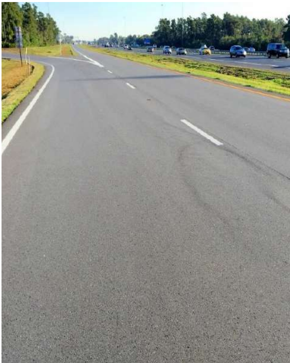
(a) Slippage at Location 1
