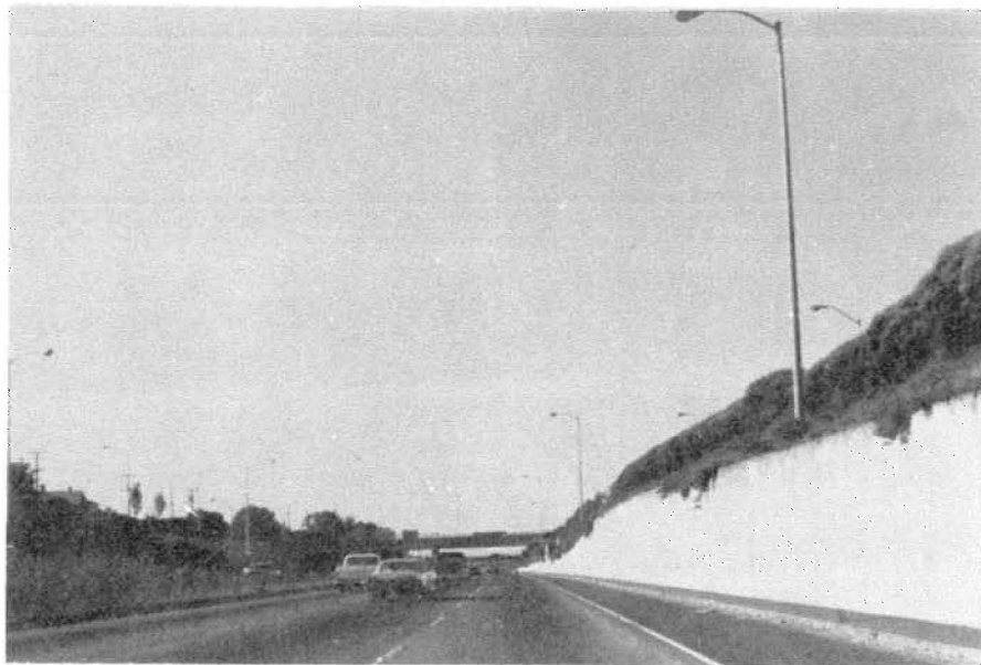
Figure 27. Luminaire supports mounted on retaining walls.
