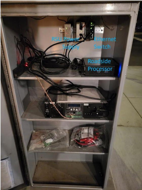
Figure 9 CV Equipment inside the Backpack Cabinet
