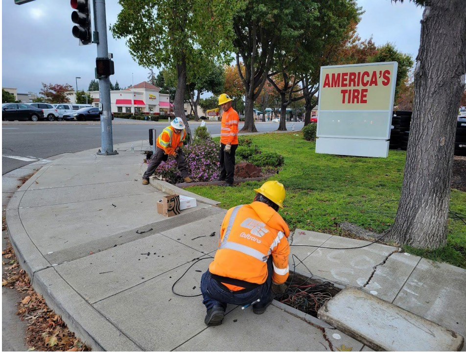
Figure 6 Pulling PoE Cable through the Conduit (From left to right: Jared Pulido, Emanuel Hernandez, and Daniel Bu)
