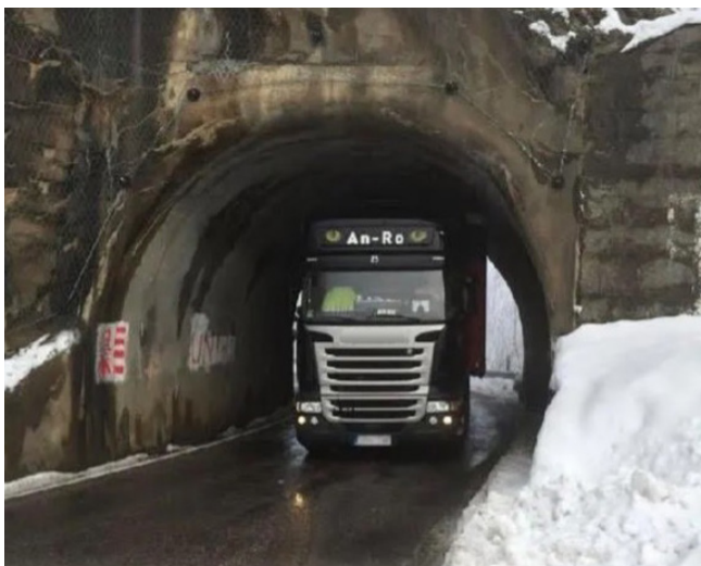
A. Before rehabilitation.
