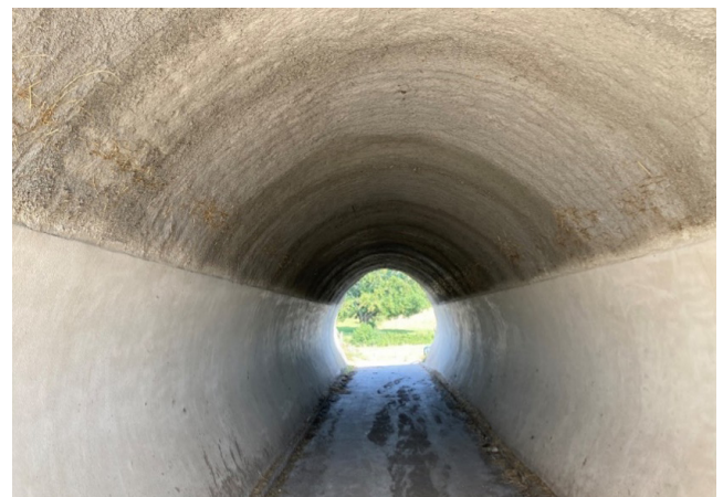
Figure 3. Photo. Interior view of the rehabilitated RCEA culvert (Huynh, Pettit, and Derimay 2019).
