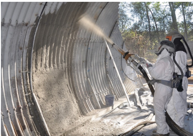
Figure 2. Photo. Spraying UHPC on the interior of the RCEA culvert (Huynh, Pettit, and Derimay 2019).
