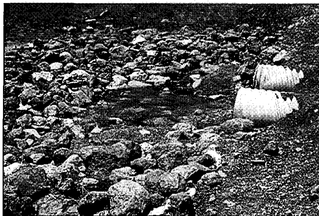
Figure 48. An encased rock berm, Round Cienega, Apache-Sitgreaves National Forests. Note exposed geotextile fabric, foreground.
