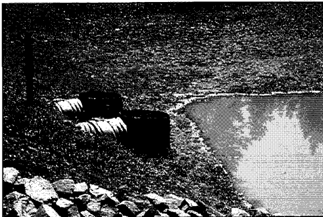
Figure 51. The potential effectiveness of these 90° elbows was negated by seepage piping through a loosely compacted embankment.
