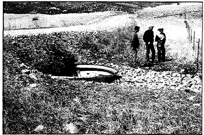
Figure 56. A drop inlet structure fashioned of steel multiplate arch, Apache-Sitgreaves National Forests.
