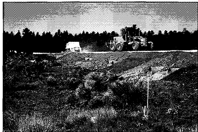
Figure 3. Improved designs are being installed in the reconstruction of Forest Road 49, Cibola National Forest, by the Federal Highway Administration.
