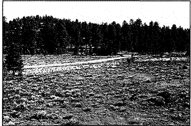
Figure 44. A completed permeable rock fill embankment, June 1995, Capulin Canyon, Cibola National Forest.
