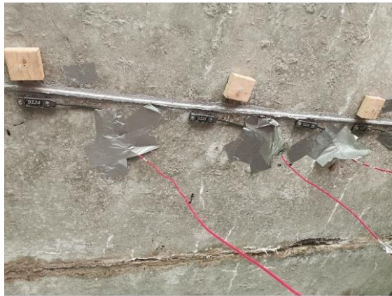
Sensors on the bottom of the slab 2
