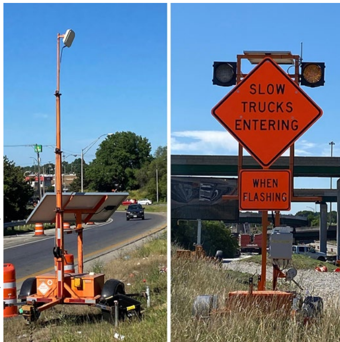
The Ohio DOT is deploying queue detection systems and flashing signs at construction exits for its I-70/71 project in downtown Columbus.
