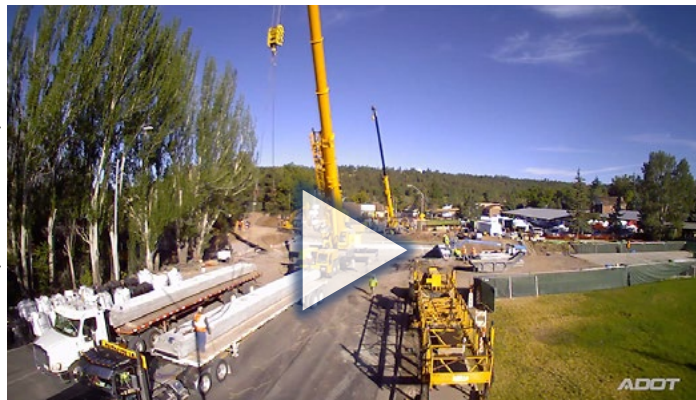
This time-lapse video shows Arizona DOT's use of prefabricated elements to accelerate replacement of a 1930s-era bridge on Route 66.
