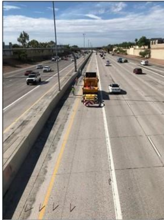
Figure 31. Setting Up Traffic Control at the Victory Drive Site and Traffic Counters Installed on a Pole
