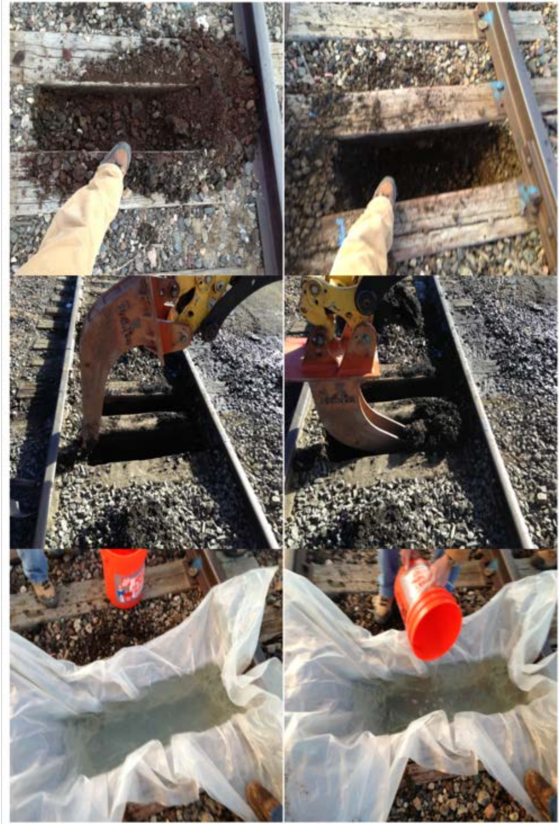
Figure 25. Ballast Sampling and Volume Measurement at Rocky Siding in CO with the Ballast Condition (Top), Excavator (Middle), and Volume Measurements (Bottom)
