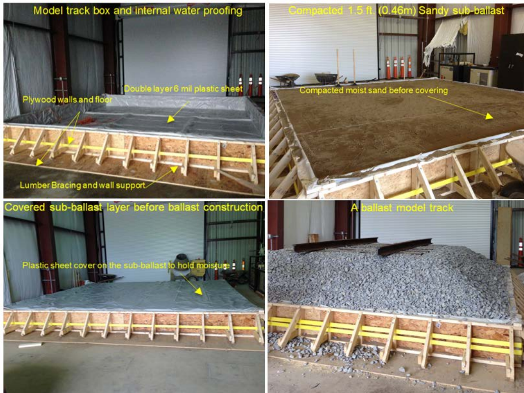
Figure 5. Photos Showing the Construction of a Ballast Model with the Lined Box for the Sub-Ballast (top left), Filled Sub-Ballast Box (Top Right), Filled and Lined Sub-Ballast (Bottom Left), and Complete Model (Bottom Right)
