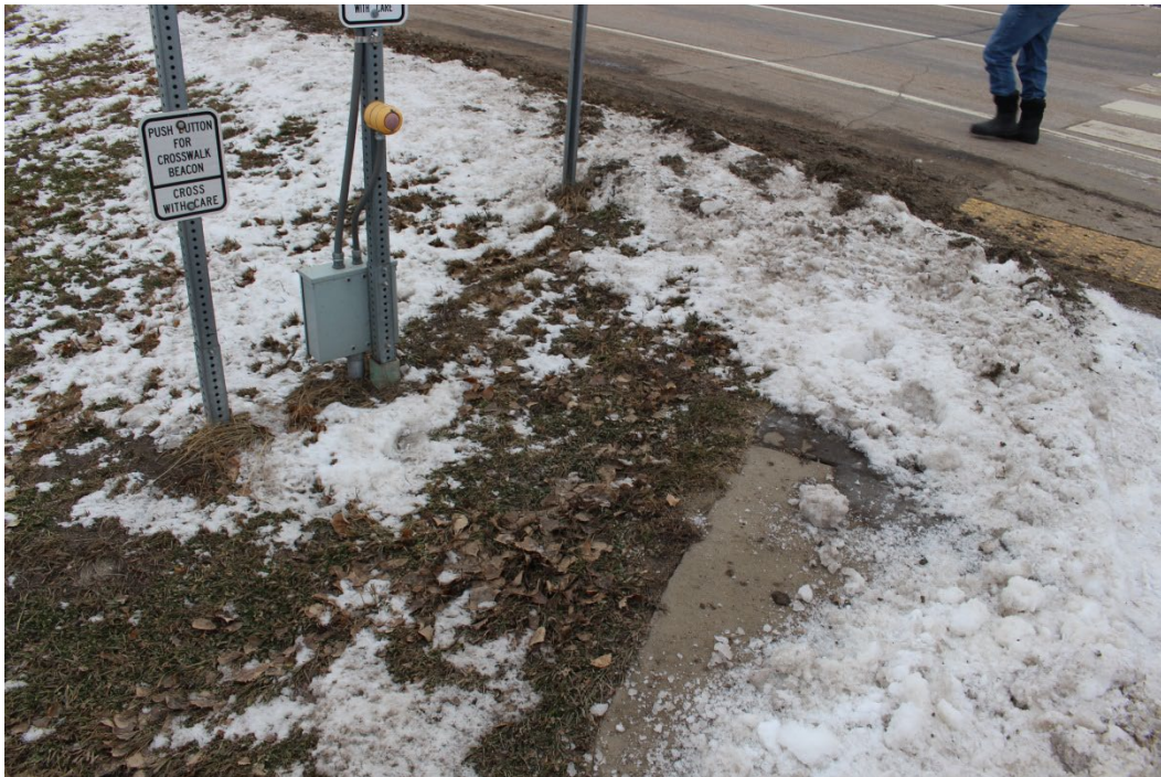
Figure 5.10 A location missing landing for the pedestrian push button
