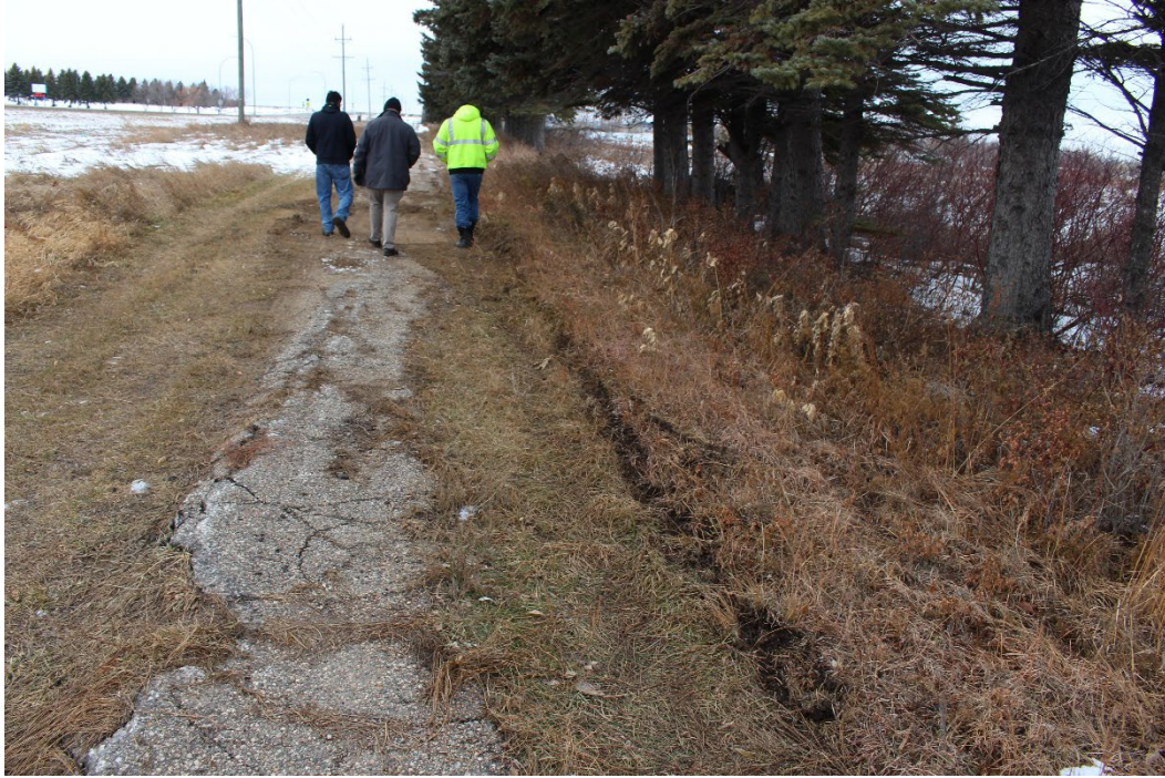
Figure 5.9 Weathered sidewalk and weeds
