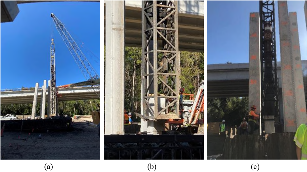
Figure 3-14. Pile driving process at Site B: (a) beginning, (b) pile at final penetration depth, and (c) driving hammer during the installation of the prestressed concrete test pile.
